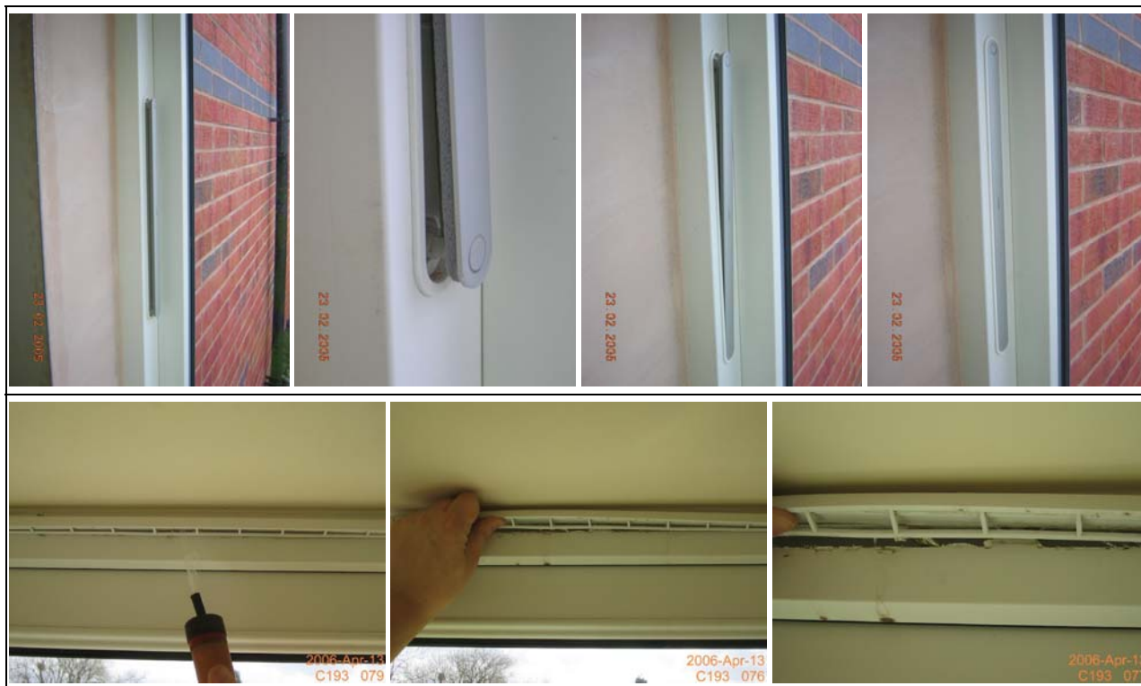
Figure 10 High performance trickle vents with compressible seals fitted at Stamford Brook (top) compared with a typical, significantly less airtight example observed during this project (below).
