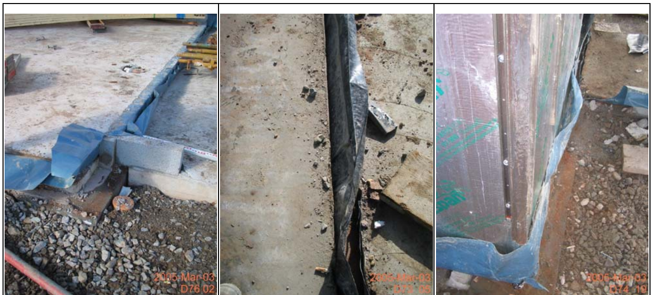
Figure 18 Developer D, Phase 3, using sacrificial blockwork to form the slab; after the blockwork is removed a straighter and more uniform slab edge reduces the potential for air leakage at this junction.
