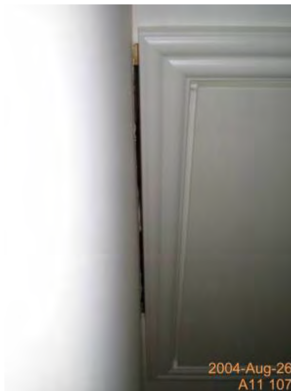
Figure 33 Loft hatch not adequately sealed to the ceiling.
