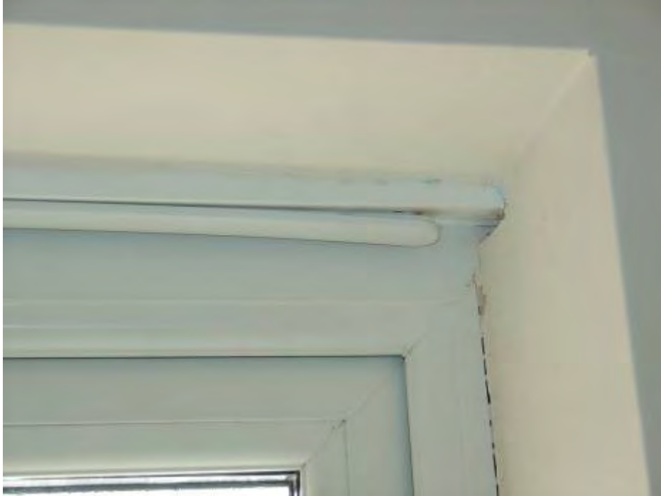
Figure 13 Leaks around poorly fitting trickle vents.
