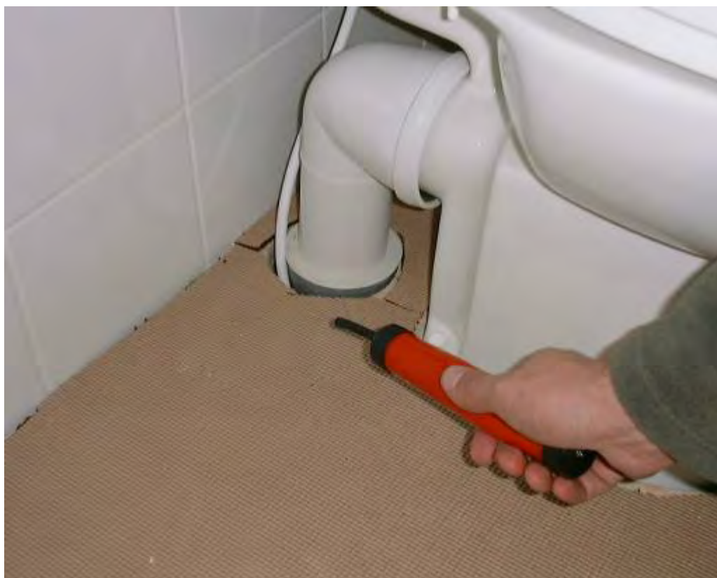
Figure B6 Leakage through service penetrations in the first floor bathroom of Plot A.
