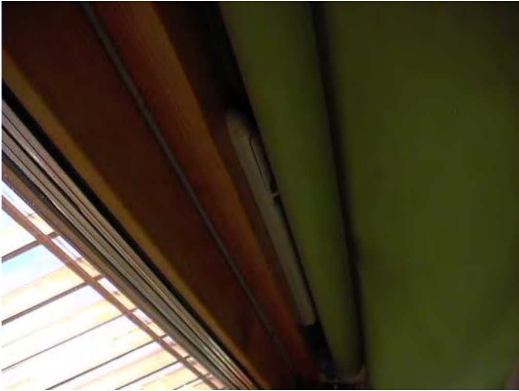
Figure B1 Leakage around trickle ventilator.
