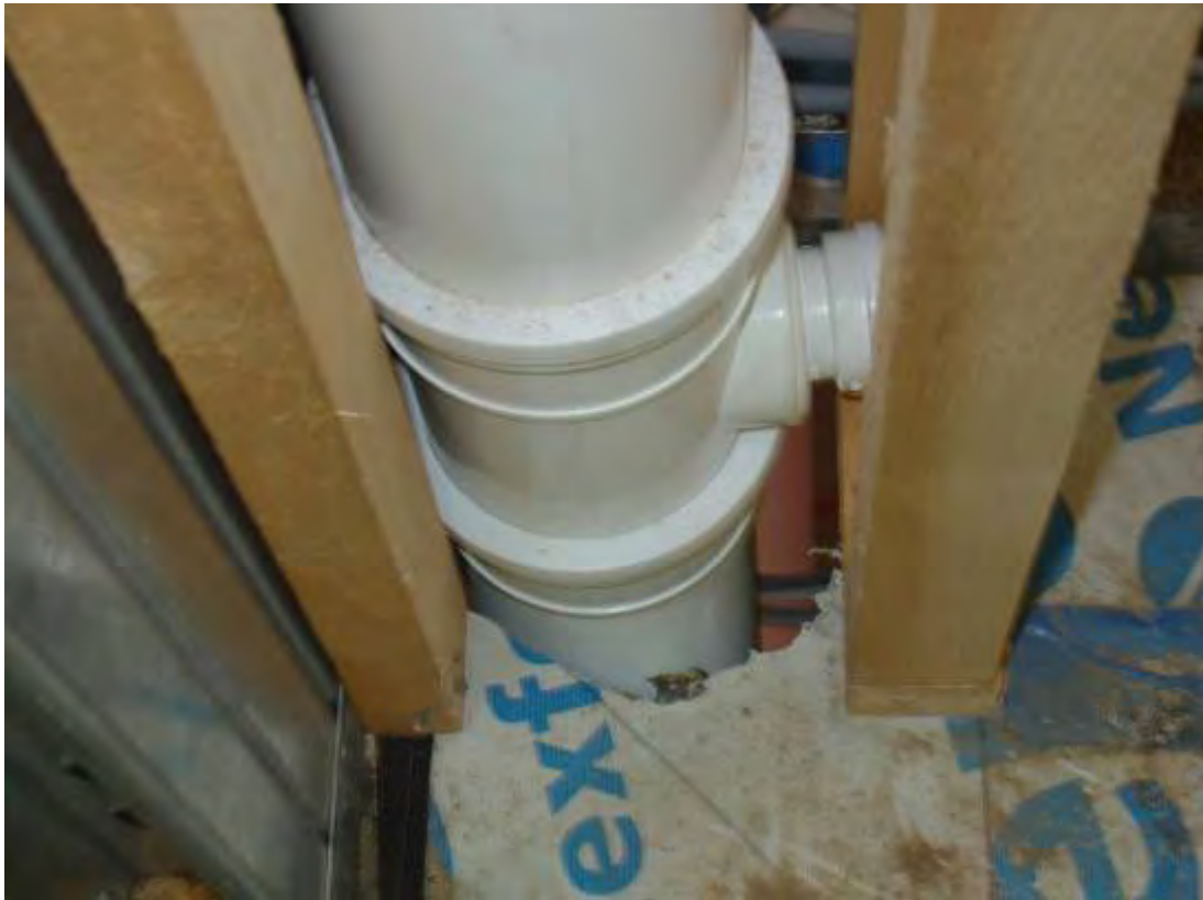
Figure 14 Unsealed soil stack penetrating through intermediate floor.
