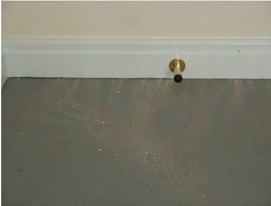
Figure 19 Dust illustrating the leakage paths at the junction between the skirting board and the first floor.
