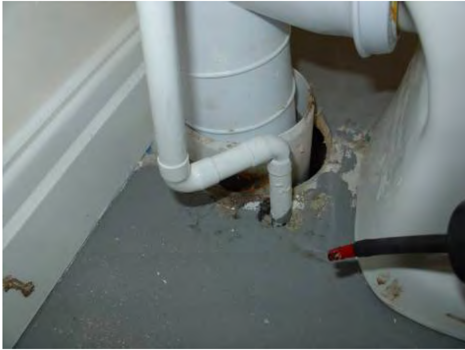
Figure 23 Leaks around water and waste pipes to toilet.
