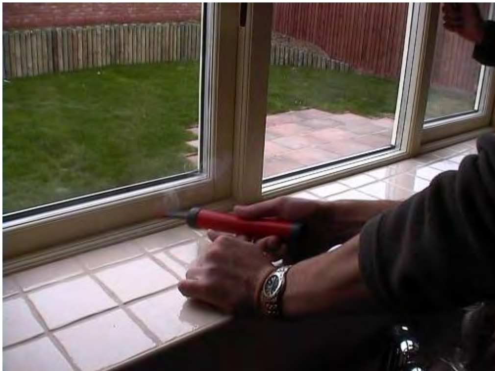
Figure B2 Leakage through opening casement in window.
