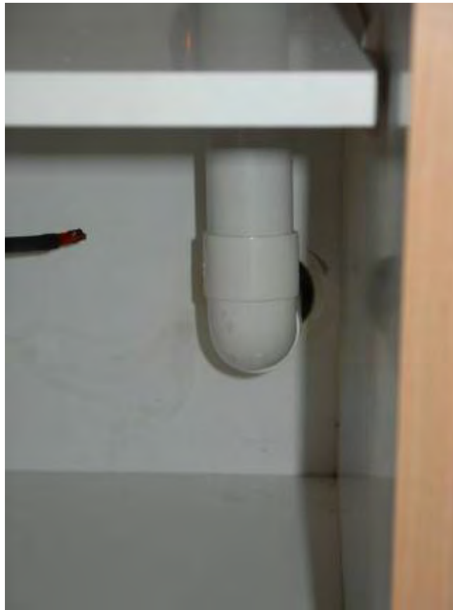
Figure 6 Leak around waste pipe.
