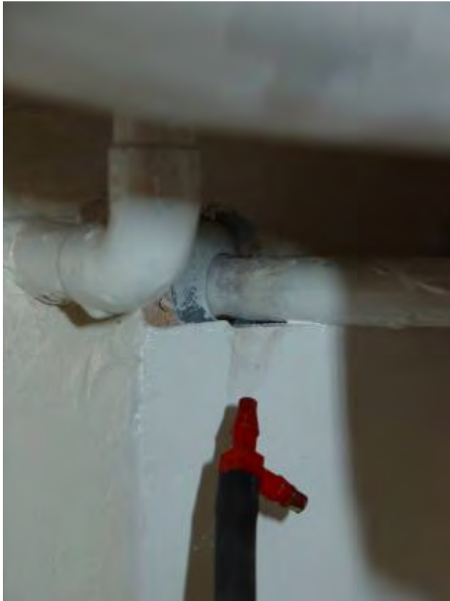
Figure 9 Leaks around water pipes to wash hand basin.
