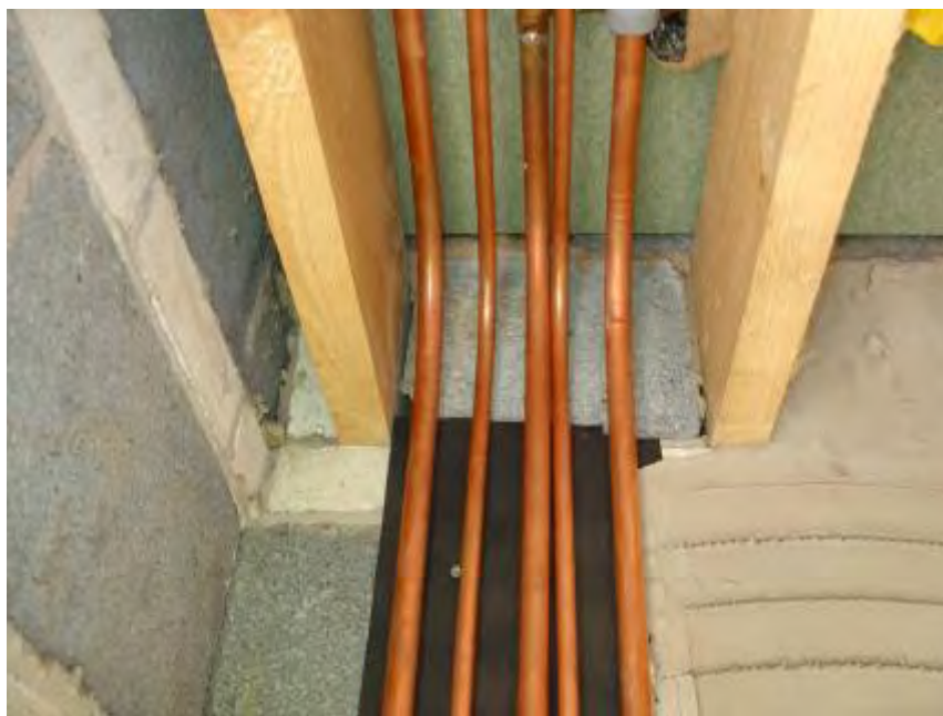
Figure 6 Incomplete scratch coat applied to party walls around services.
