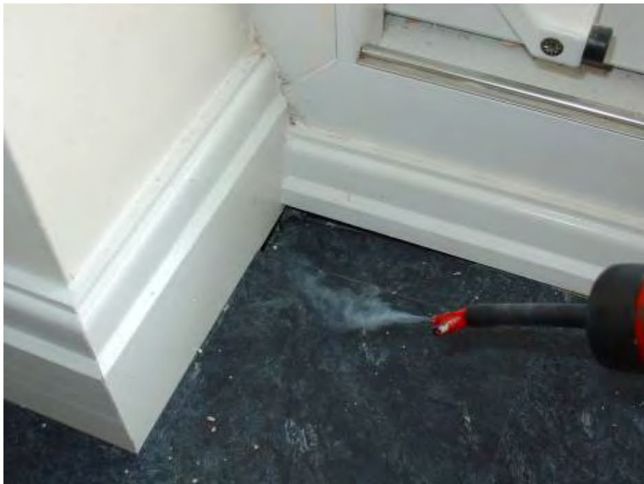
Figure 12 Leak at hole in kitchen floor.
