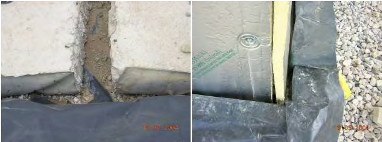
Figure 17 Developer D, Phase 1, the use of removable polystyrene formers created an inconsistent and uneven slab edge, with potential for air leakage at the junction of slab, steel frame and insulation.
