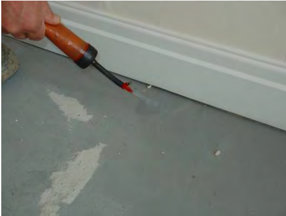
Figure 4 Leak at gap between skirting board and floor.
