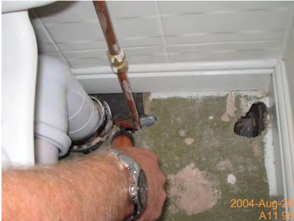
Figure 22 Holes in bathroom floor.
