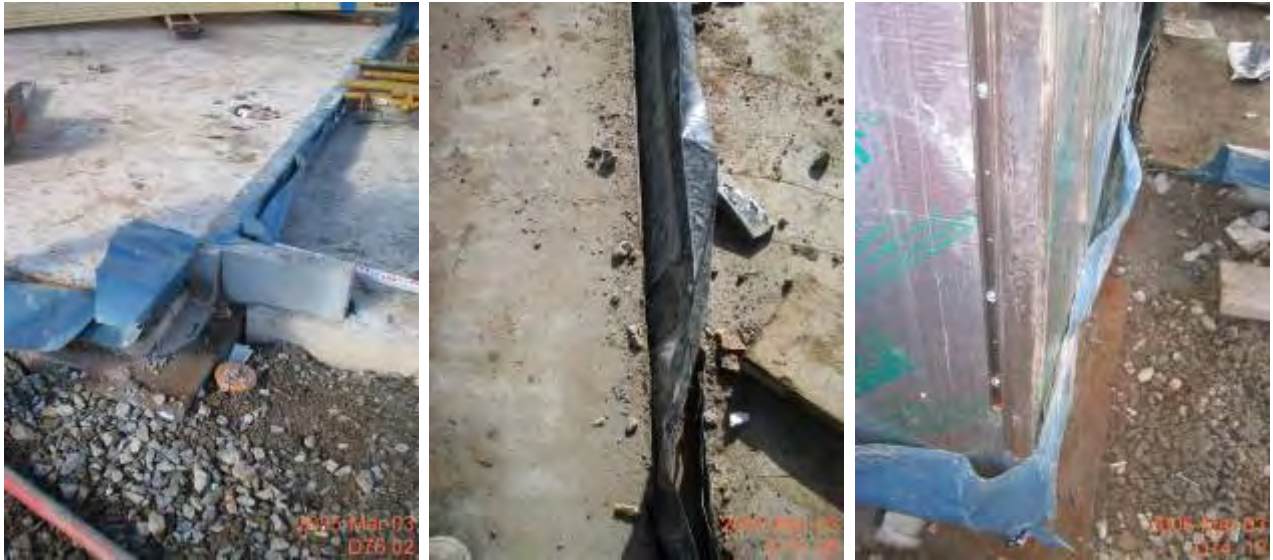
Figure 18 Developer D, Phase 3, using sacrificial blockwork to form the slab; after the blockwork is removed a straightener and more uniform slab edge reduces the potential for air leakage at this junction.
