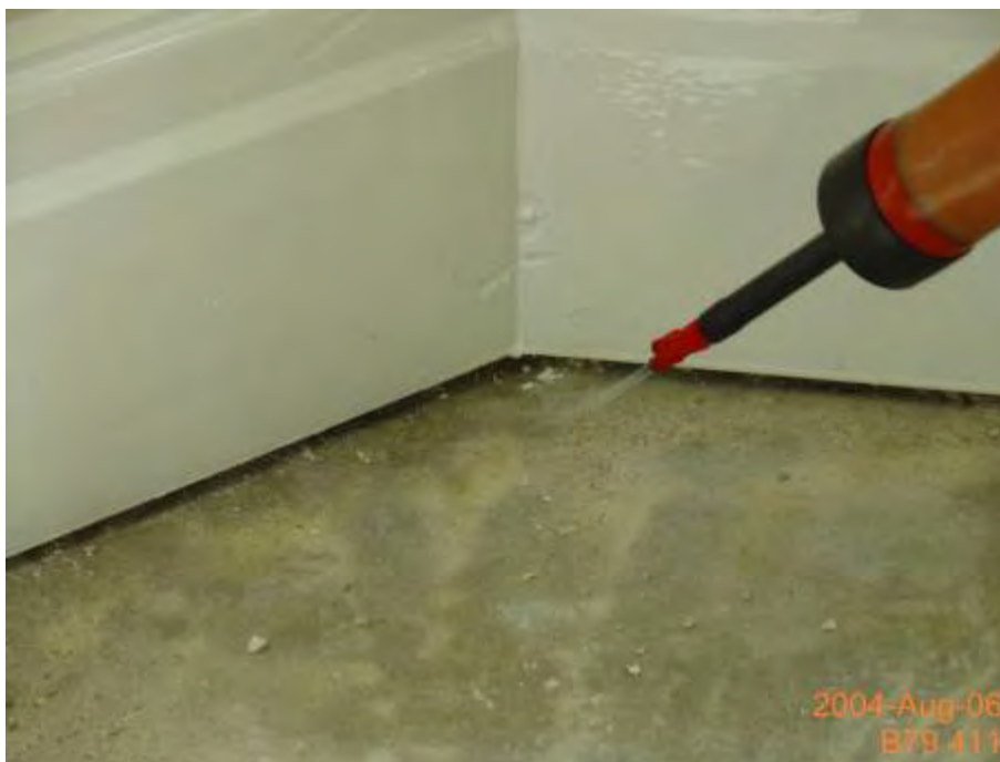
Figure 28 Leak at gap between skirting board and ground floor.
