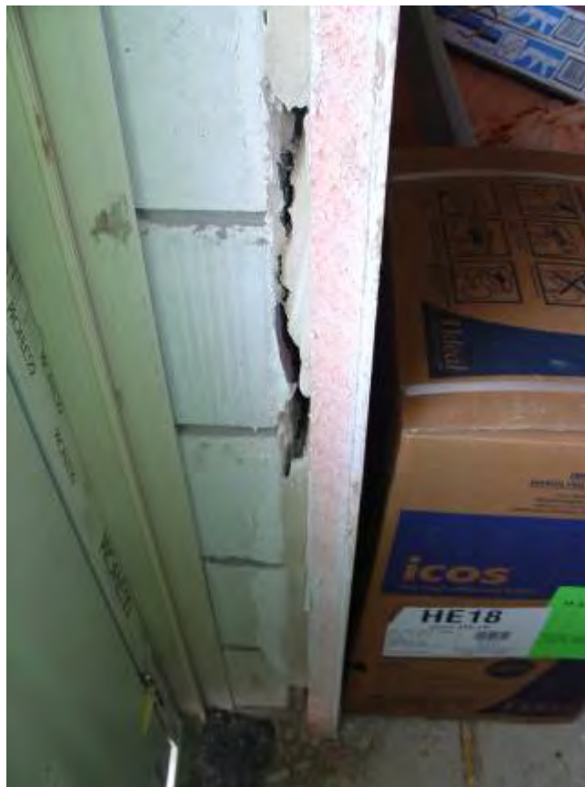
Figure 11 Discontinuous ribbons of adhesive around door opening.
