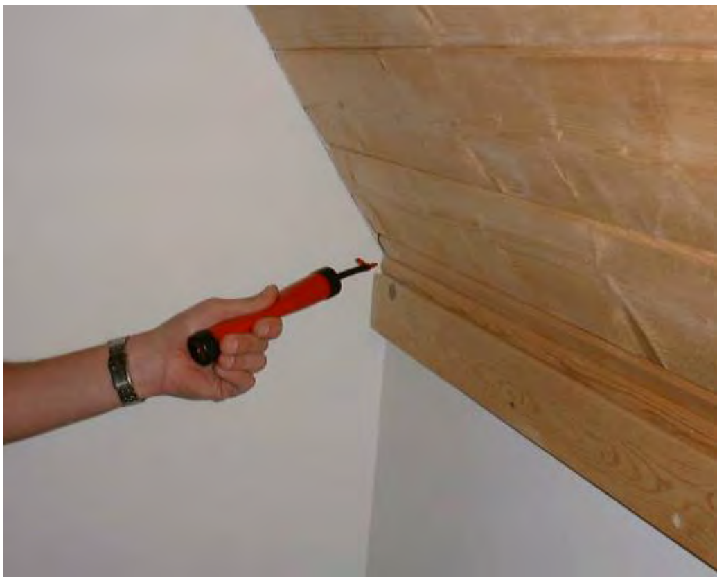
Figure B2 Leakage at junction between the ceiling and the internal and external walls.
