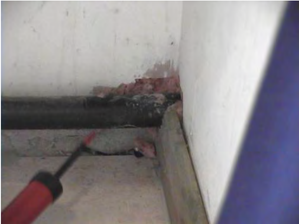
Figure B3 Leakage through service penetration in kitchen.
