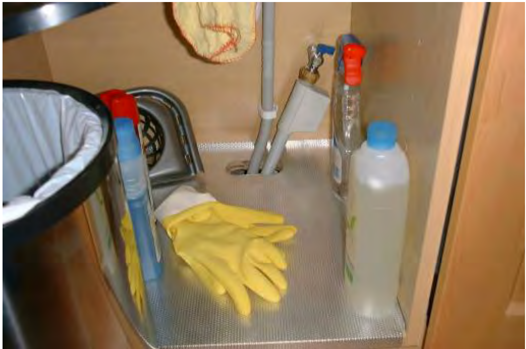
Figure B4 Leakage through service penetrations in the kitchen of Plot A.
