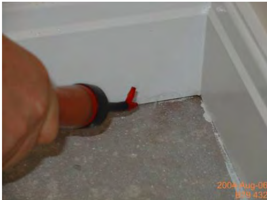
Figure 30 Gaps at the junction between the skirting board and the first floor.
