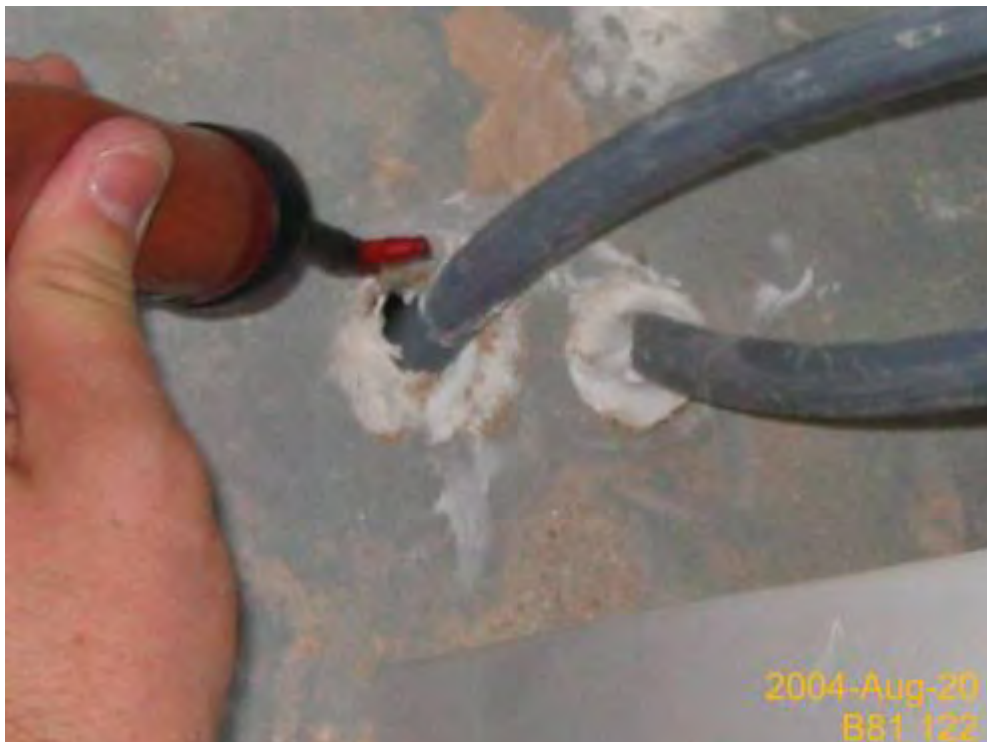
Figure 16 Unsuccessful attempt at sealing around water pipes.
