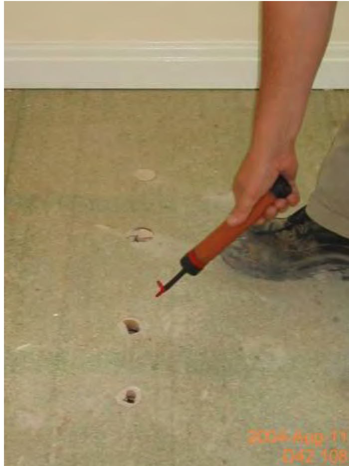
Figure 20 Holes in the flooring panels.
