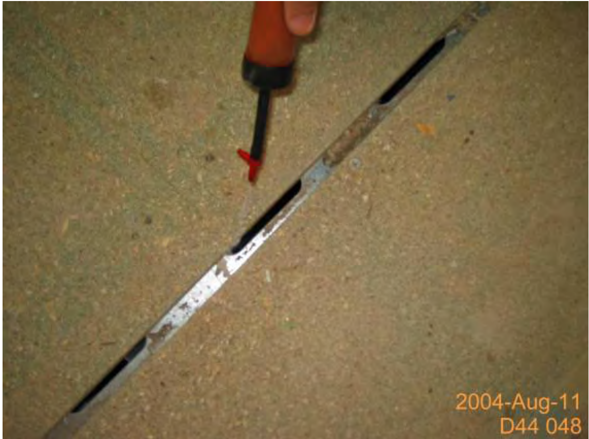
Figure 19 Leaks at the junction between flooring panels.
