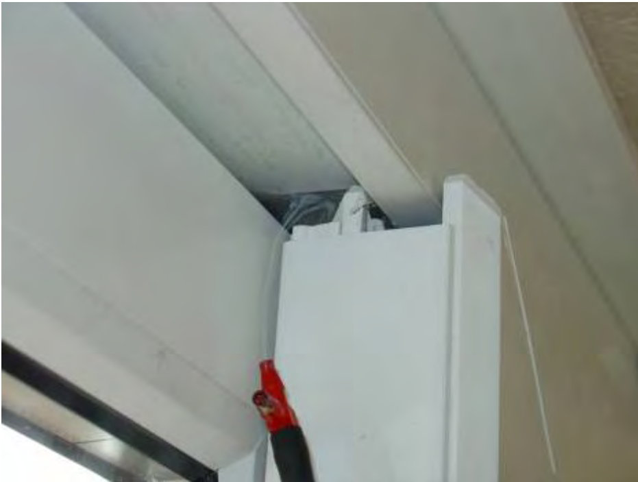
Figure 14 Leaks around junction at top of patio doors.
