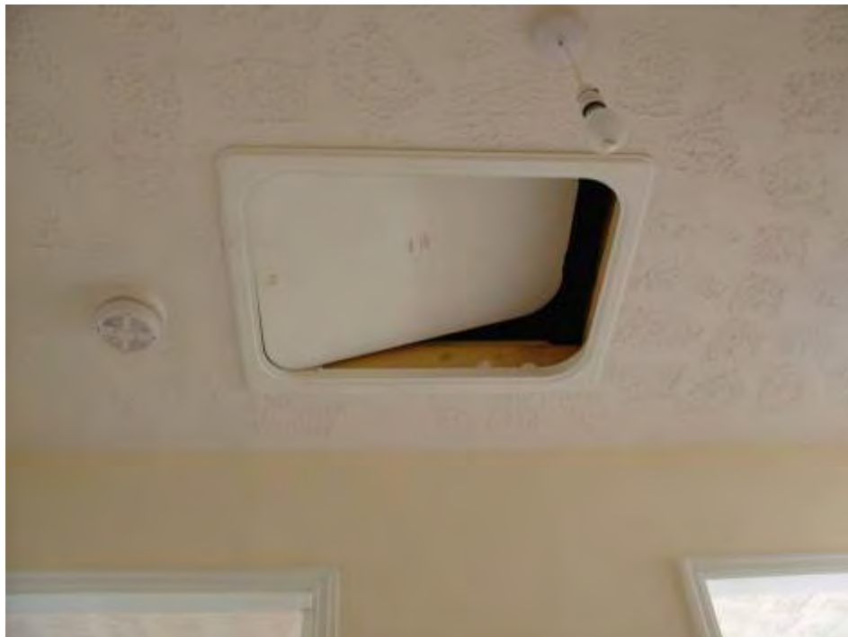
Figure 18 Poorly locking loft hatch lifting during leakage identification.
