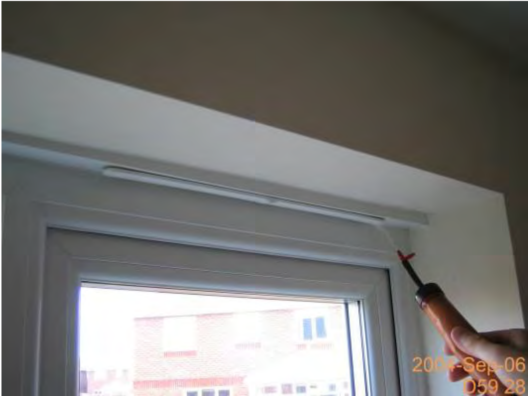
Figure 25 Leakage through poorly fitting trickle vents.
