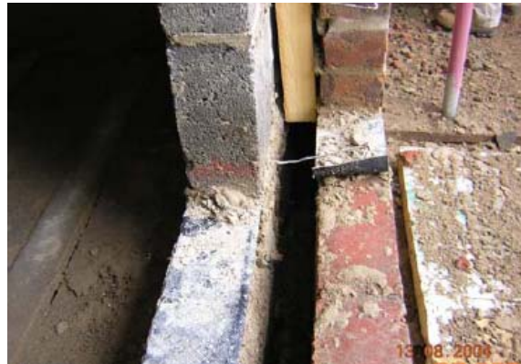
Figure 3.11 Perimeter insulation missing below dpc in masonry construction.
