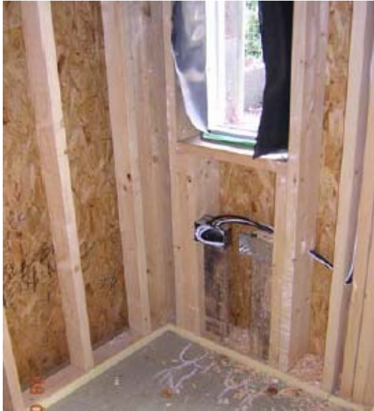
Figure 3.79 Small gap between studs (also, note high timber concentration at corner).
