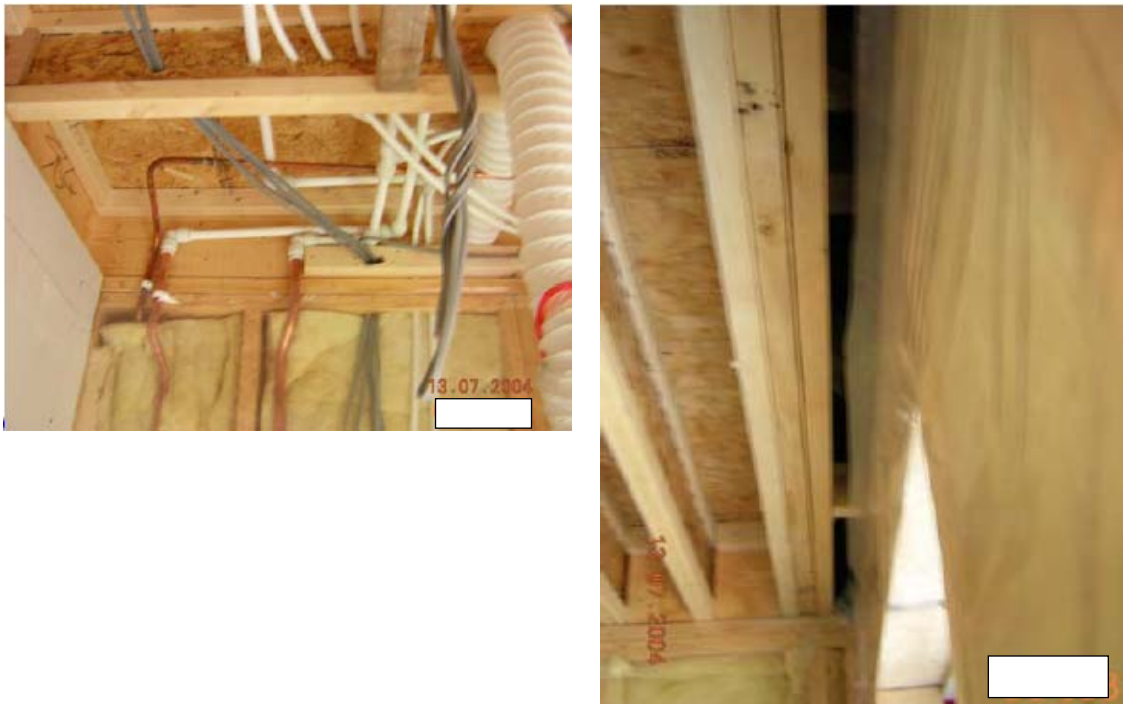
Figure 3.25 High concentration of services and close proximity of I-beam to external wall reduce both access and the likelihood of effective insulation at intermediate floor perimeter.
