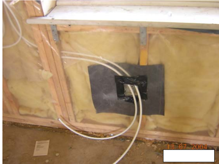
Figure 3.87 Air/vapour control layers not lapped to DPC 1 .
