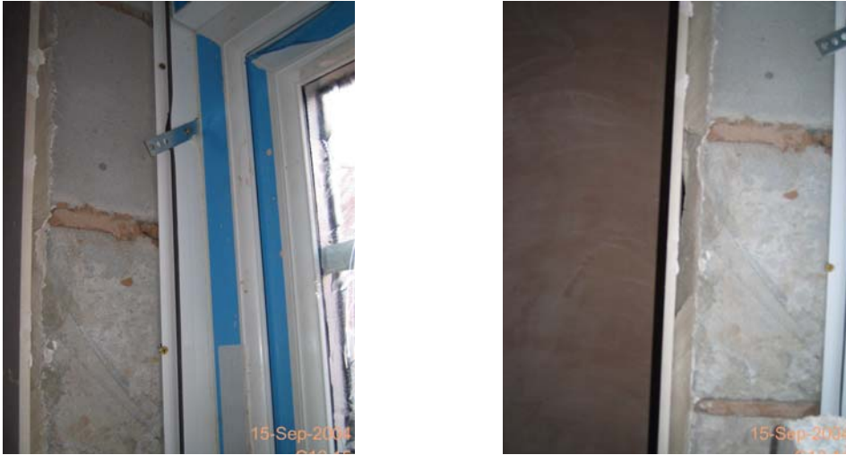
Figure 3.92 Continuity of plaster adhesive - an unusual case.
