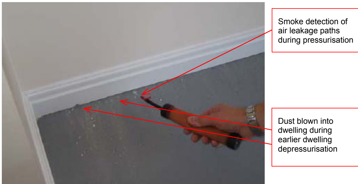
Figure 3.29 Air leakage through intermediate floor junction (Johnston et al, 2004).
