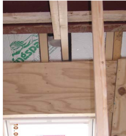
Figure 3.52 Gaps around insulation boards between rafters.
