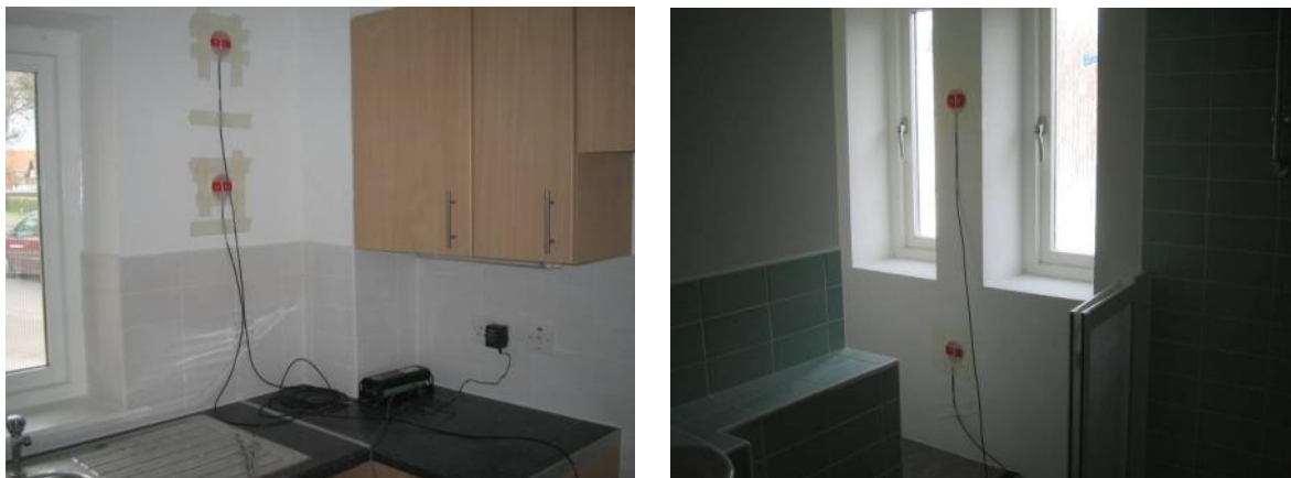
Figure 31 – Heat Flux Sensors on North Facing Wall of Kitchen and Top Floor Bathroom
