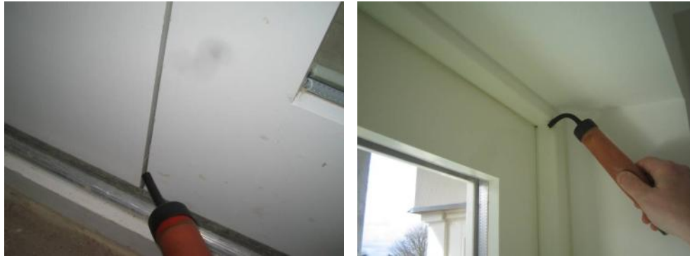
Figure 28 – Leakage at Door and Window Seals
