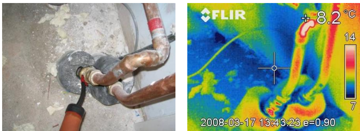
Figure 23 – Leakage at Heat Main Floor Penetration using Smoke and Thermal Imaging
