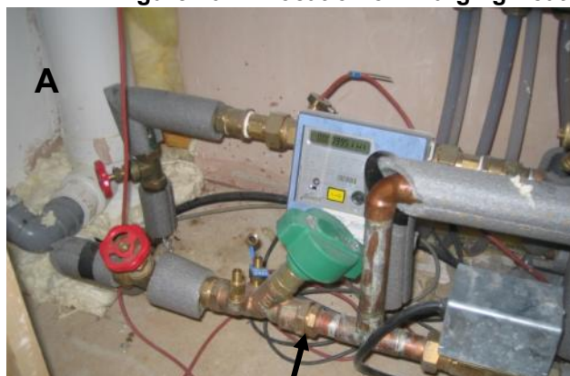
Missing Temperature Sensor before Hot Water Split
