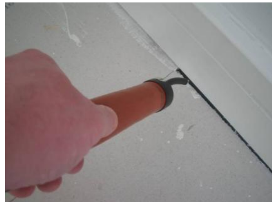
Figure 17 – Leakage via Floor-Wall Junction
