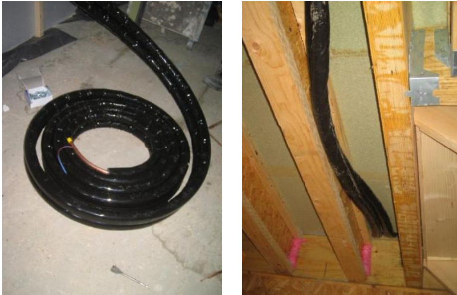
Figure 14 – Solar System Pipework
