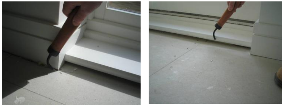
Figure 29 – Leakage at Thresholds
