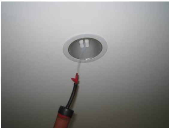
Figure 16 – Leakage via Recessed Light
