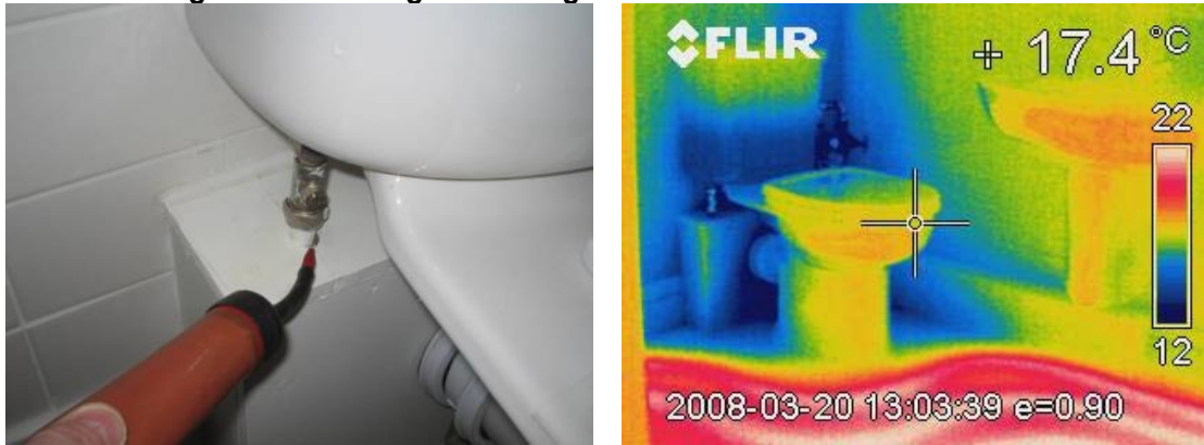
Figure 24 – Leakage at Boxing-in around Toilet on Ground Floor
