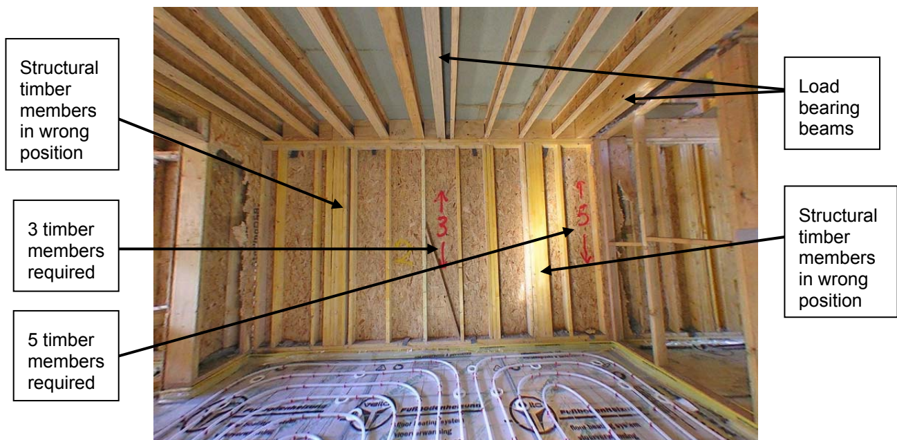
Figure 59 – Photograph of Exposed Party Wall Panels Showing Missing Structural Members
