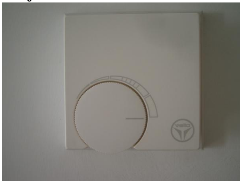
Figure 123 – Room Thermostat Dial at Elm Tree Mews
