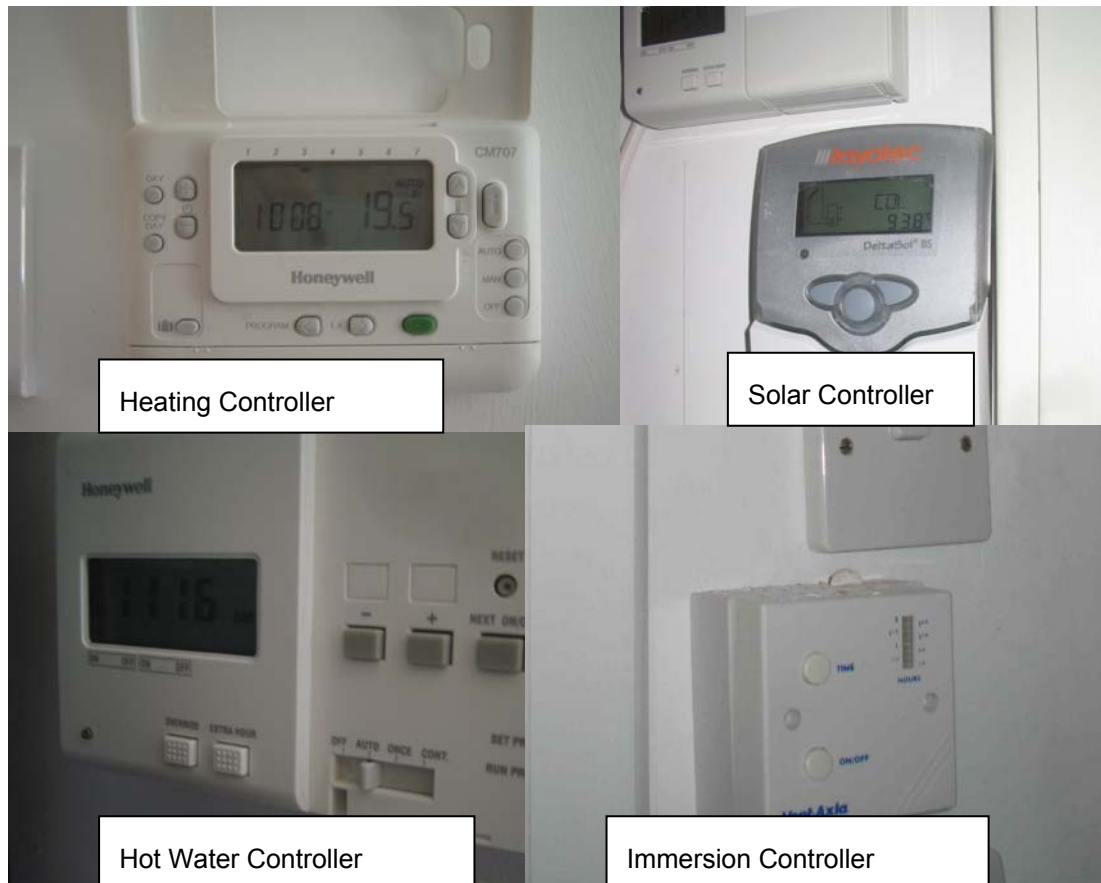
Figure 122 – Heating System Controls
