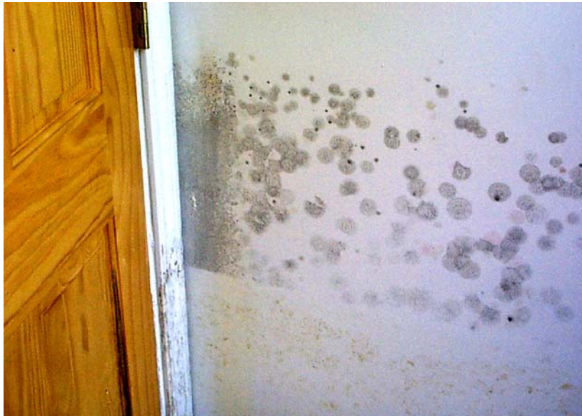
Figure 6 - Interior Plasterboard Showing Surface Mould Growth after a Flood Test (ORNL 2005)
