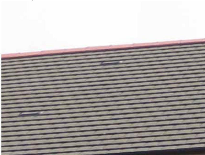
Figure 6 – Low Profile Roof Tile Vents on Plots 405 and 406
