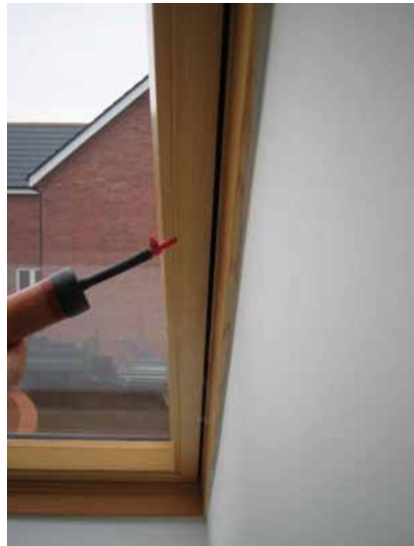
Figure 56 - Leakage at Rooflight Seal
