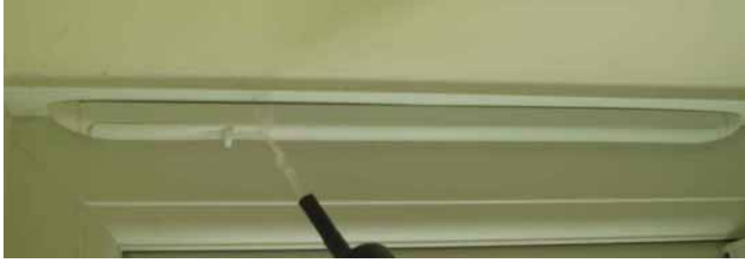
Figure 48 - Leakage around Typical UK-sourced Trickle Vent (picture from Leeds Met L2 project)
