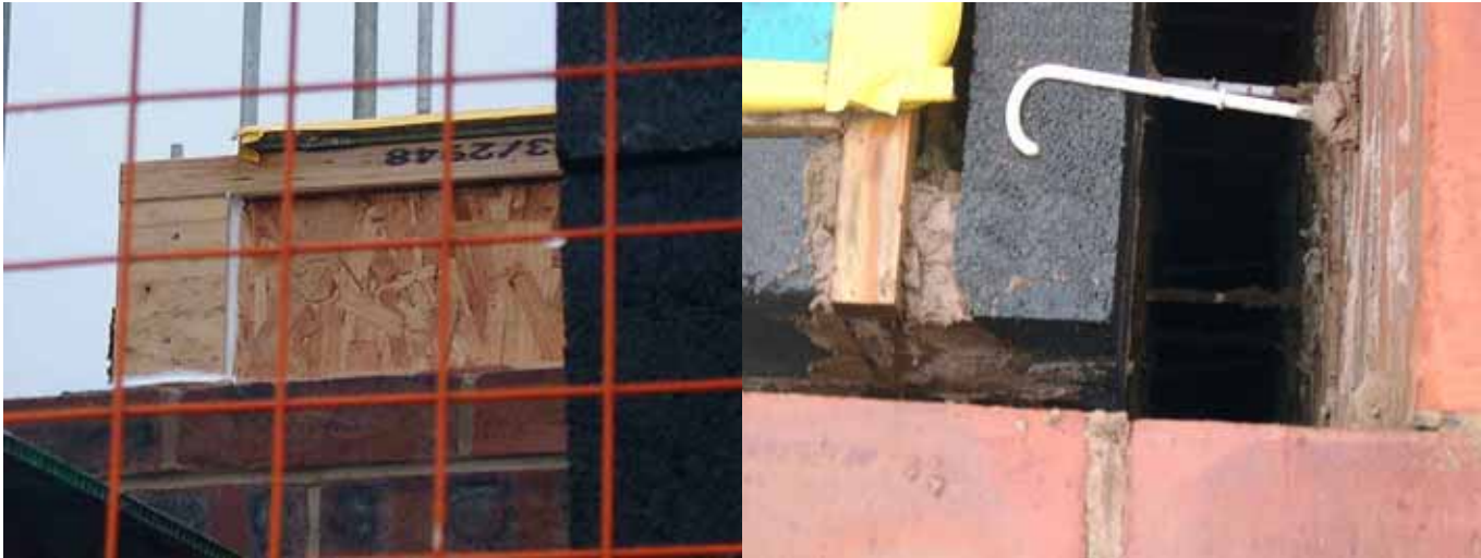
Figure 91 Filler End Pieces on I-beam Web Figure 92 Gap Filled between End Beam and Wall
