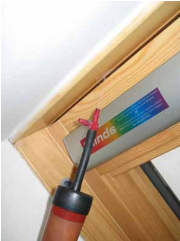
Figure 55 - Leakage at Rooflight Seal
