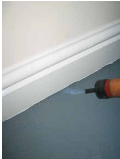
Figure 73 - Leakage at Floor-Wall Junction
