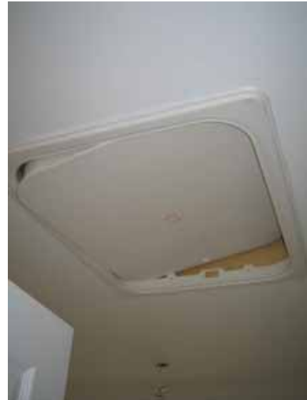
Figure 60 - Hatch Dislodged during Test
