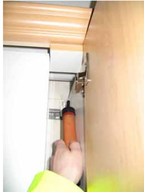
Figure 64 - Leak behind Kitchen Cabinets
