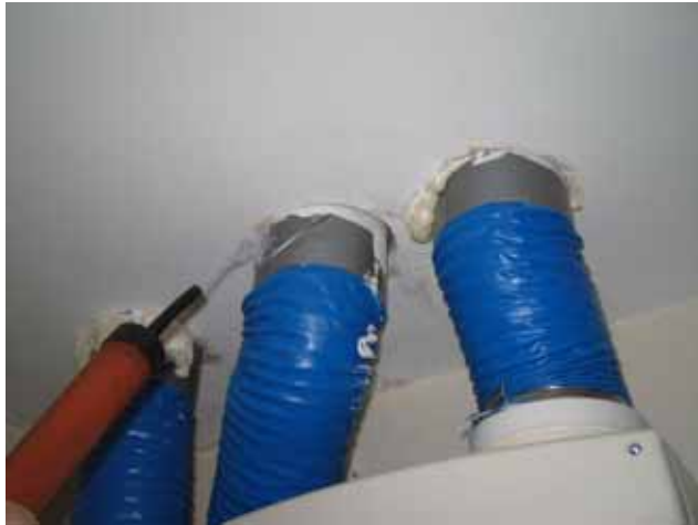
Figure 71 - Unsealed Duct Penetration
