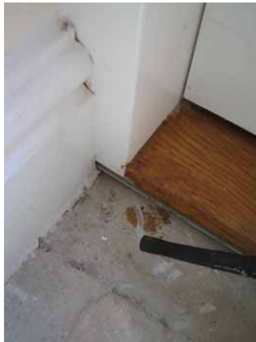
Figure 50 Patio Door Leak at Threshold Corner
