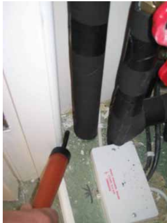
Figure 70 Leak at Wall-Floor Junction in Cupboard
