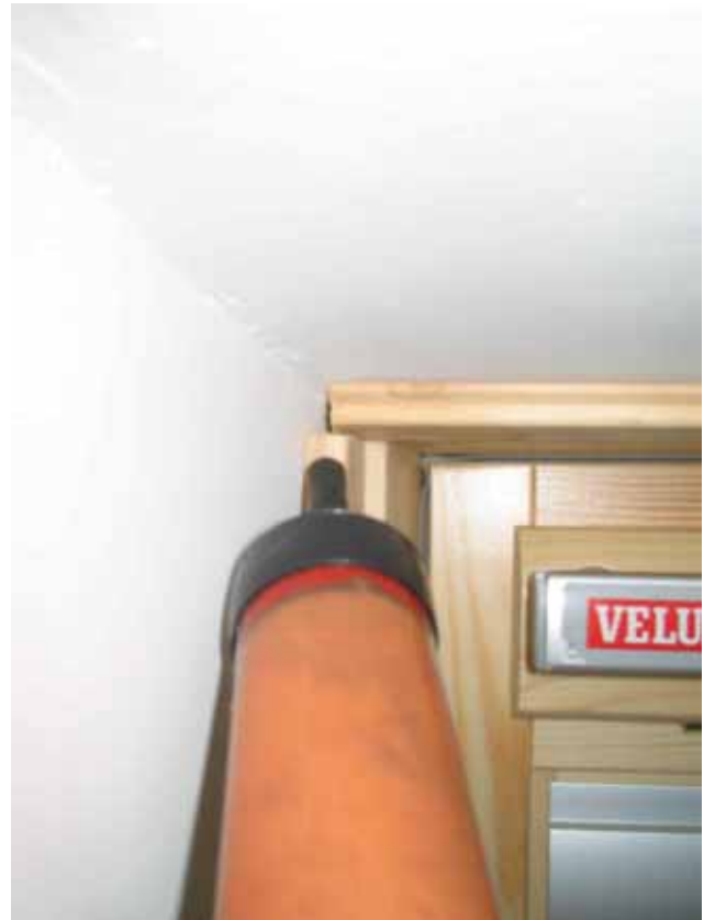
Figure 54 - Leakage around Rooflight Frame
