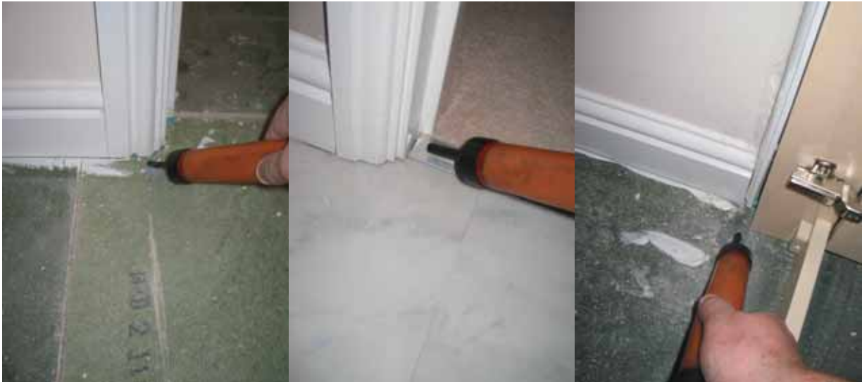
Figure 75 - Leak at Partition Wall Figure 76 - Leak at Partition Wall Figure 77 - Leak at Partition Wall
