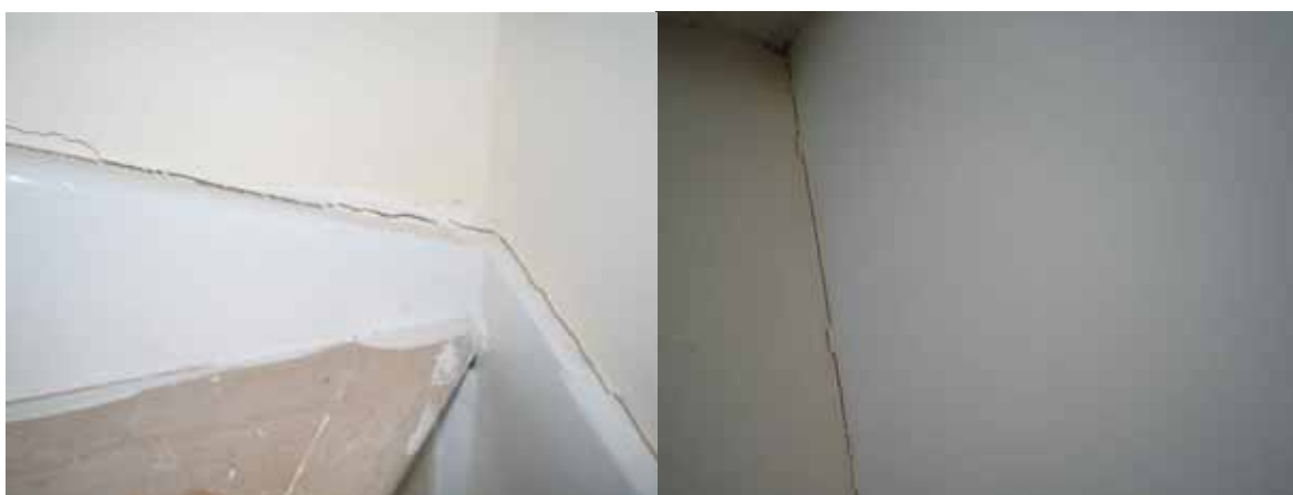
Figure 10 - Cracks in Internal Walls of Plot 402 following Co-heating Test
