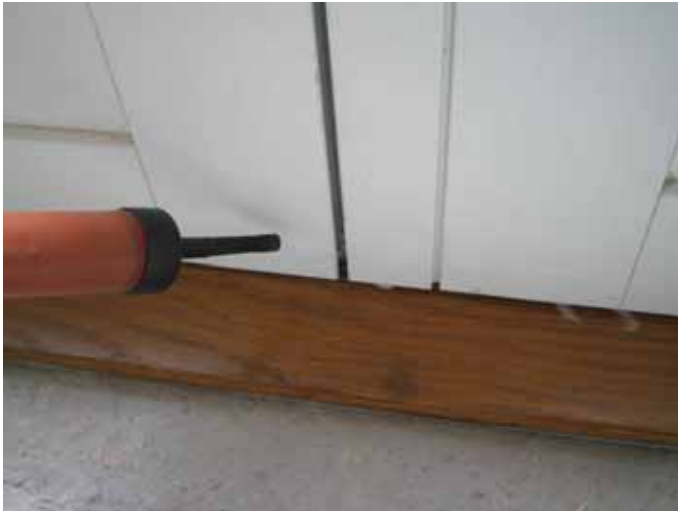
Figure 51 - Leak between Patio Doors
