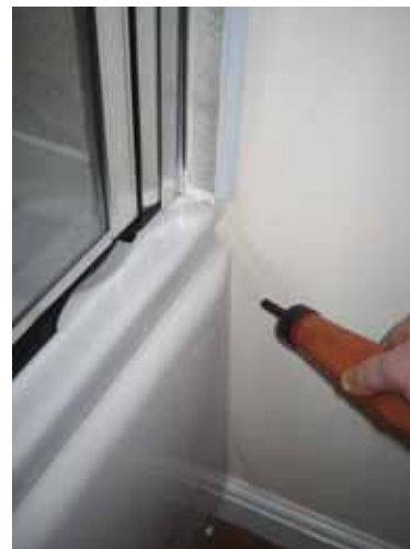
Figure 62 - Leak at Shower Tray
