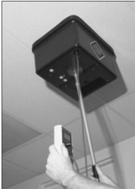
Figure 98 - Exhaust Fan Flow Meter in Operation (Energy Conservatory 2003)
