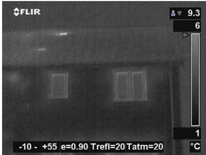
Figure 105 - Thermal Image Showing Heat Loss at MEV System Roof Terminal Vent
