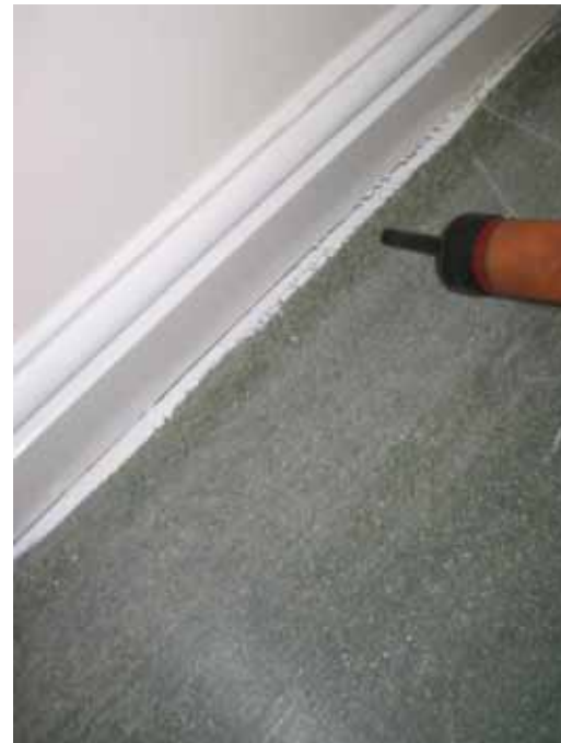
Figure 74 - Leakage at Floor-Wall Junction
