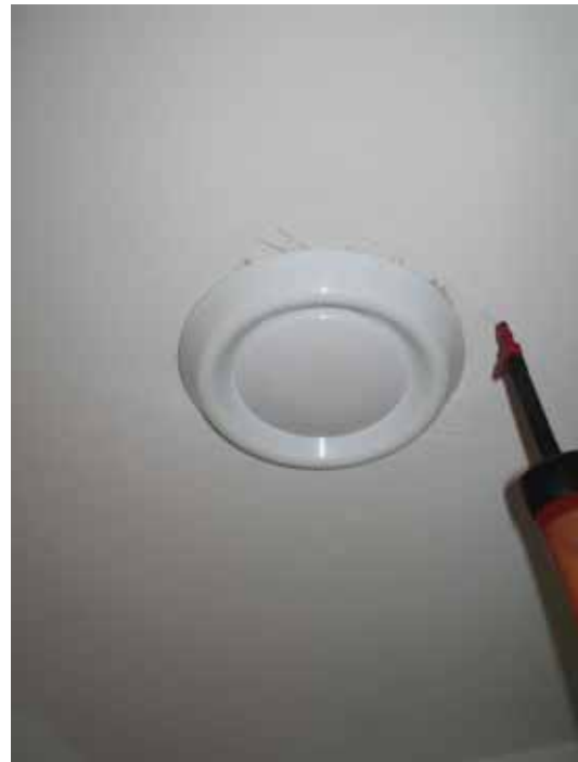
Figure 79 - Leak around MEV Extract Vent
