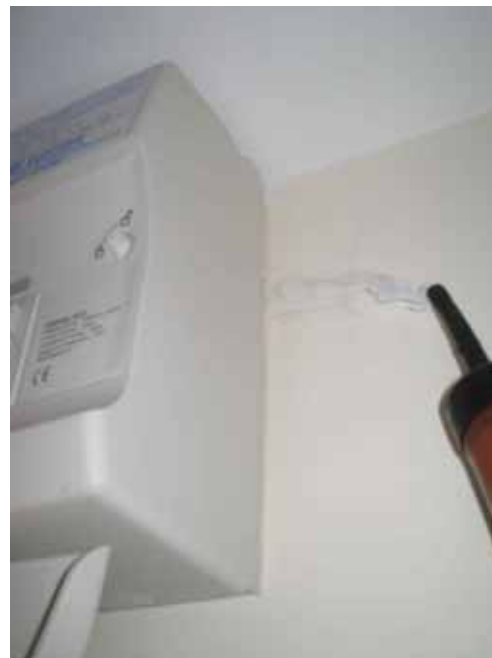
Figure 66 - Leak behind Consumer Unit
