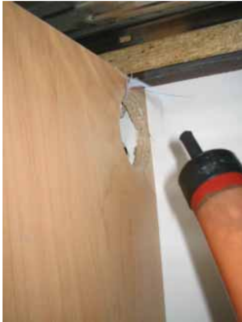
Figure 63 - Leak behind Kitchen Cabinets
