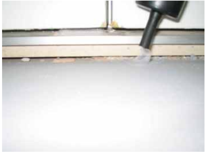
Figure 52 - Leakage under Threshold
