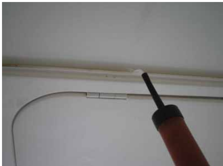
Figure 58 - Leakage between Hatch Frame and Ceiling
