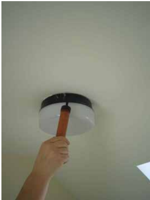
Figure 78 - Leak around Light Fitting
