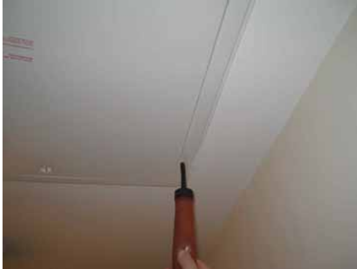
Figure 59 - Leakage between Loft Hatch and Frame
