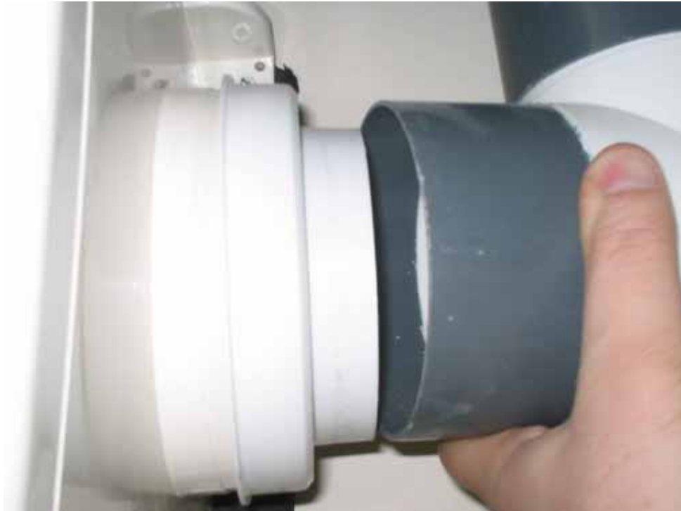
Figure 5 – Loose Spigot Connection
