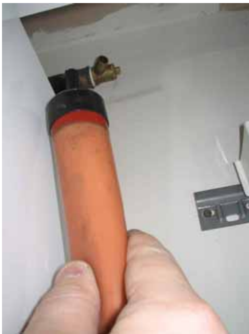
Figure 65 - Leak at Boiler flue
