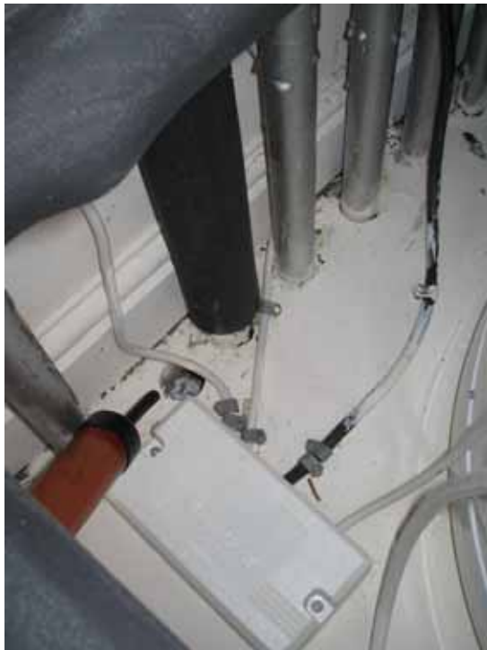
Figure 69 Leak through Unsealed Hole
