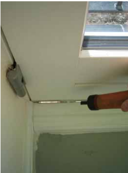
Figure 49 Patio Door Leak at Unsealed Threshold
