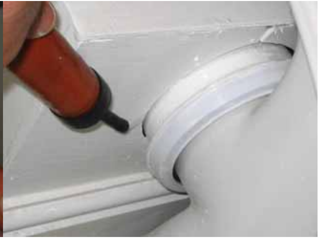
Figure 68 - Leak where Toilet Soil Pipe enters Boxed Service Void
