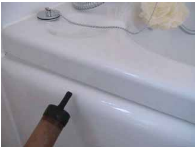
Figure 61 - Leak around Bath Panel
