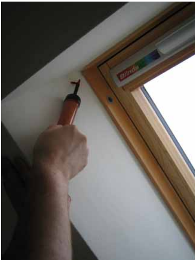
Figure 53 - Leakage around Rooflight Frame
