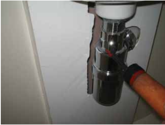
Figure 67 - Leak at Cut-out for Sink Trap
