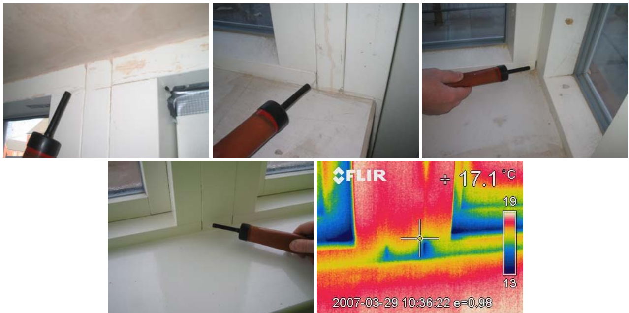
Figure 16. Air leakage through gaps at bay windows in plots B116 and R111
