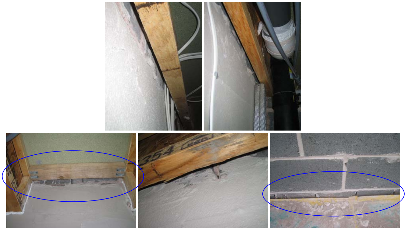
Figure 49. Examples from all of the Bryant plots studied, illustrating where gaps in the parging layer behind joists, joist struts and floor decking appear.
