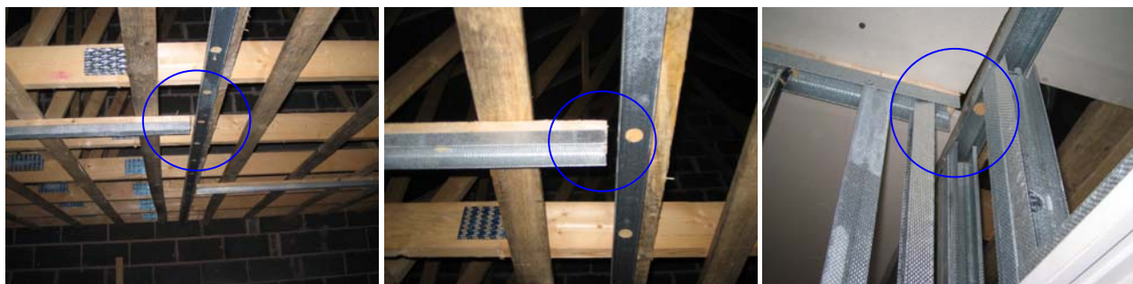
Figure 73. Gaps between timber head plates and metal studwork in plot R110.
