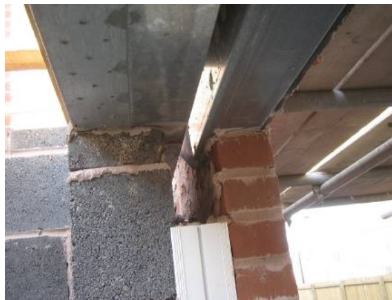
Figure 111. An incorrect window former in plot B119 leaving a gap at the jamb/head junction which was not always sealed effectively.
