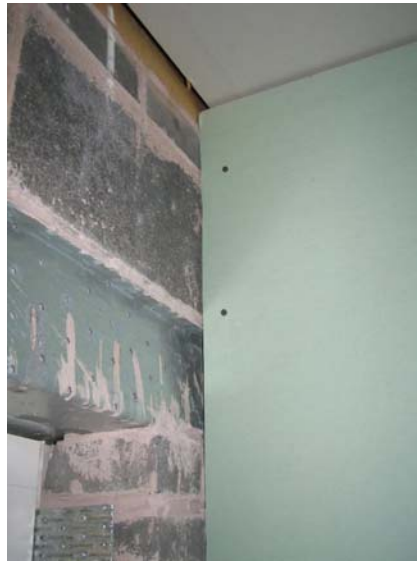
Figure 46. Erection of partitions before paring; creating an air barrier discontinuity (plot B116).
