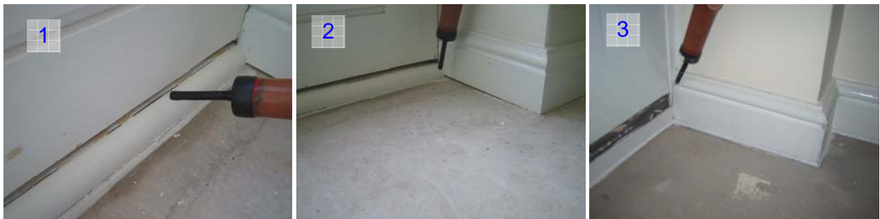
Figure 11. Air leakage at the patio door threshold in plot R110 (1 & 2) and at the threshold reveals of single leaf back door in plot B120 (3)
