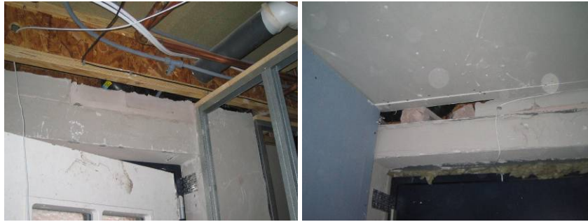
Figure 110. Recessed front door head in plot R116 with patched up blockwork after access for the soil pipe, in plot R117 the weakened repaired blockwork damaged during dry-lining.
