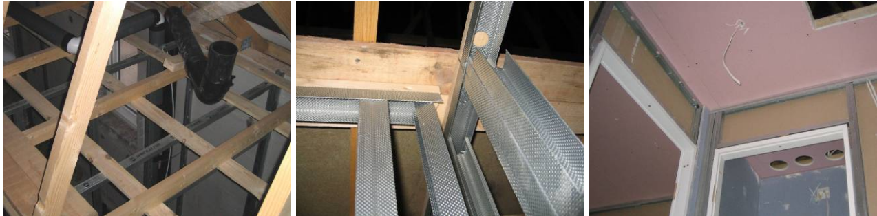
Figure 102. Open gaps in the partition head studwork in Redrow area 3; the gaps covered by timber head plates in plot R111 but with gaps still remaining at partition junctions; a full ceiling in plot B119 erected prior to the partitioning with easily sealable gaps around penetrations.
