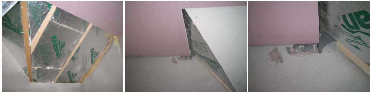
Figure 90. Sloping ceiling sections to the side of the dormer window in the XT2 and XT house types with the horizontal ceiling installed prior to the membrane in sloping sections.
