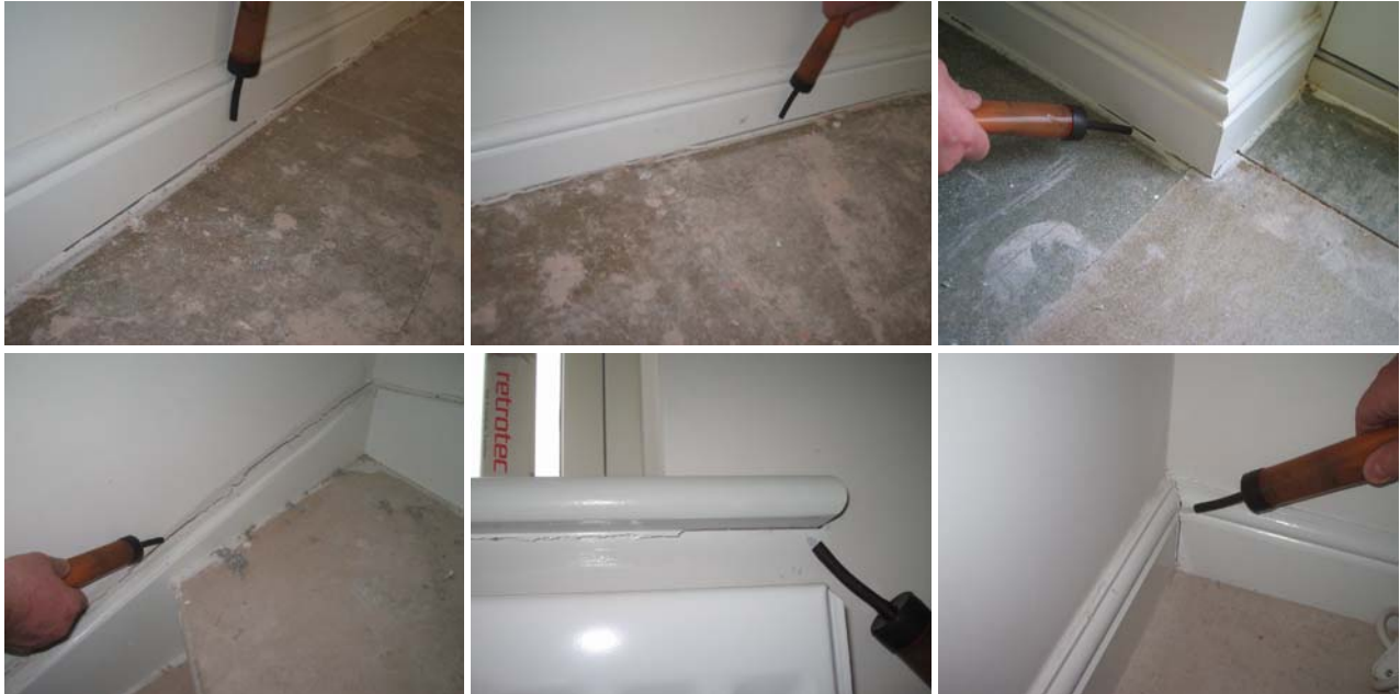
Figure 99. Air leakage detected during the re-test of plot R110, through failed secondary sealing and shrinkage cracks following the co-heating test.
