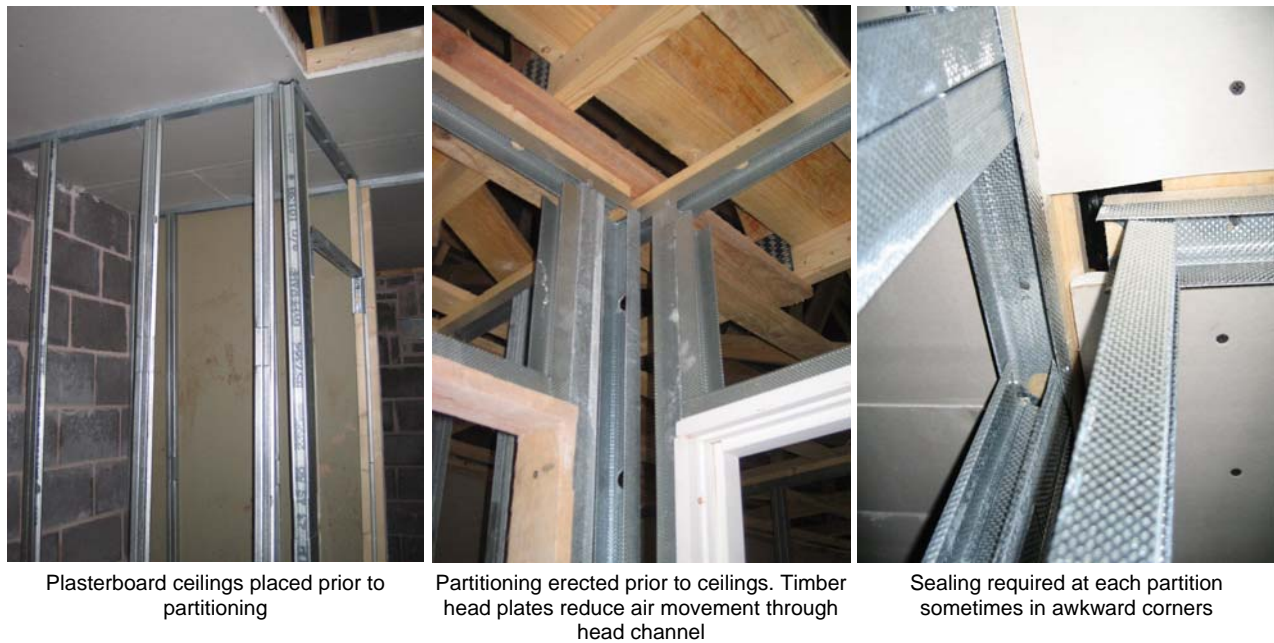
Figure 72. Full plasterboard ceilings before erection of the partition in Bryant plot B116 compared with Redrow's partitioning with timber head plate first approach in plot R111.
