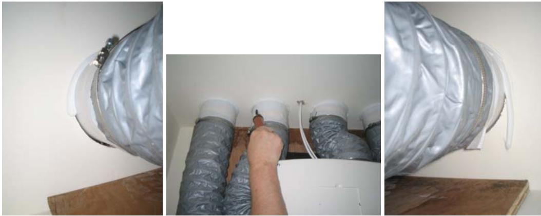
Figure 79. Gaps in the sealant and air leakage around the MEV ducting in plot B119.
