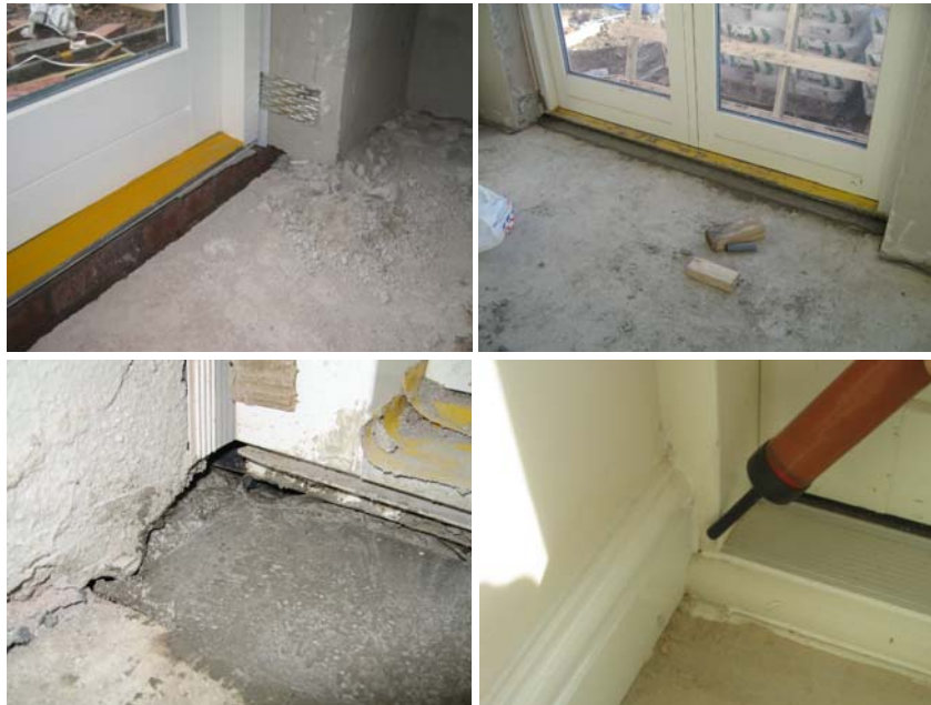
Figure 42. The patio door threshold in plot R116.
