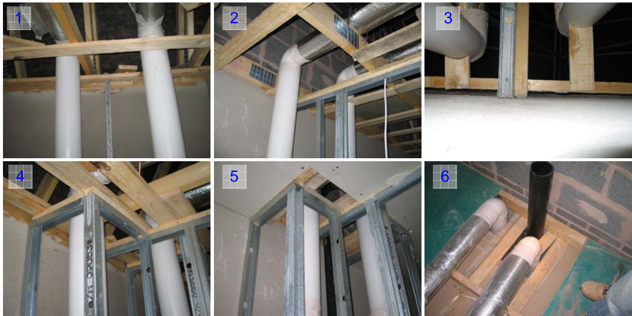
Figure 83. The service void straddling the partition wall between bathroom and bedroom in plots R110 and R111.
