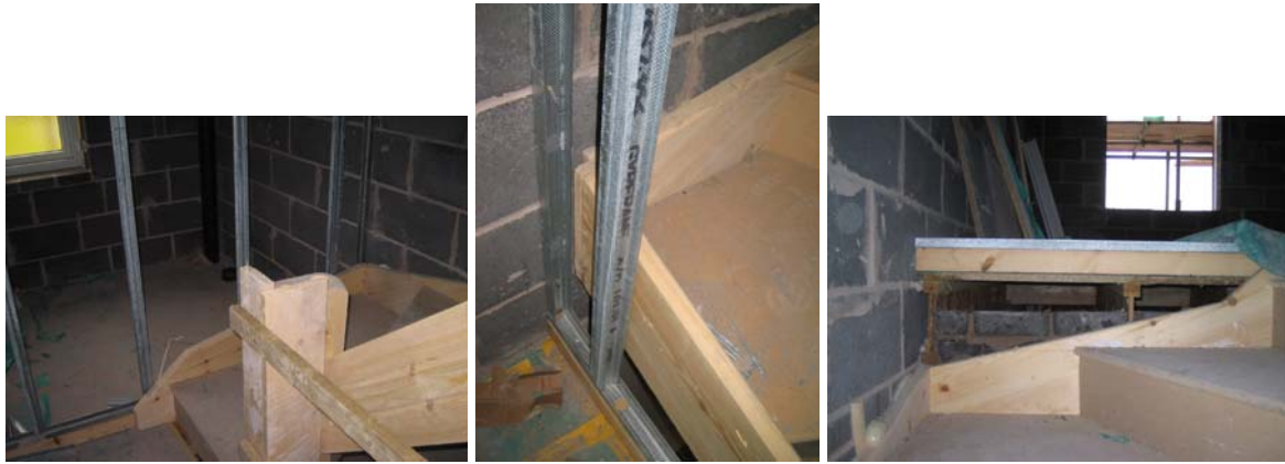
Figure 48. The staircase between the 1 st and 2 nd floors in plot R110, installed before the parging coat had been applied to the party wall.
