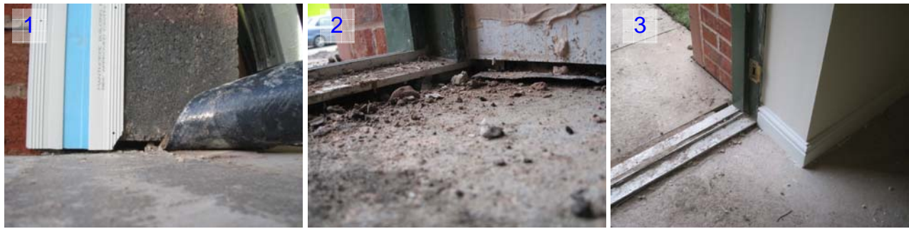
Figure 41. The front door threshold in plot R111.
