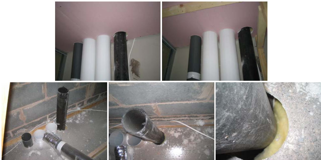
Figure 80. Penetrations through the ceiling inside the service void in the rear en-suite bathroom in plot B119.
