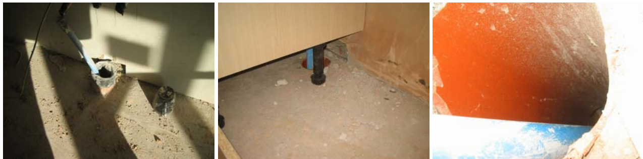
Figure 35. Mains water supply pipe in the kitchen of plot R116.
