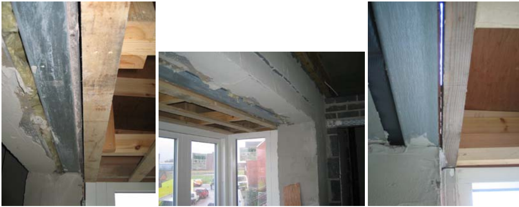
Figure 63. Incomplete parging of the lintel over bay window openings and leakage routes to the outside via the flat bay roof void.
