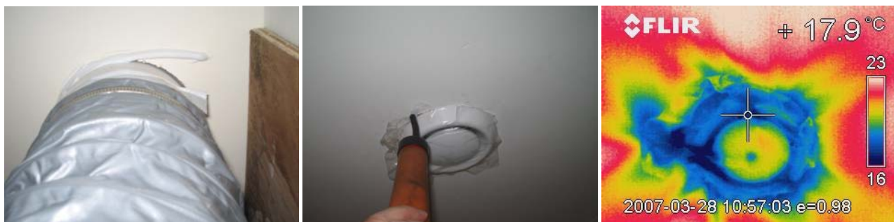
Figure 21. Ventilation ducts in B119 and vent in R110
