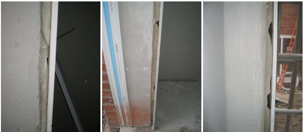
Figure 51. Photographs of plot R116, at the front door, back door and patio door; the gaps in the plasterboard adhesive ribbons are illustrative of the good, typical and poor examples observed.
