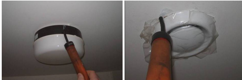
Figure 7. Detection of direct air leakage paths from the top floor bathroom of plot R111 into the attic, under dwelling pressurisation using smoke puffers.
