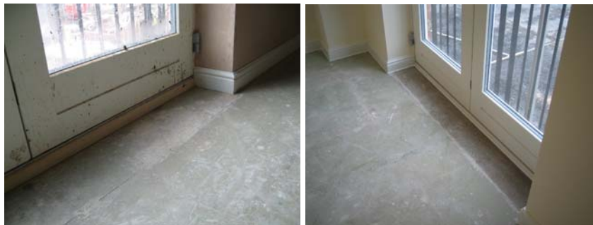
Figure 66. Balcony door thresholds with timber filler pieces inserted.
