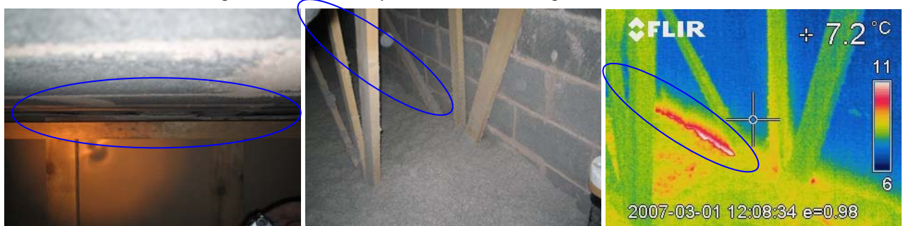
Figure 76. Images taken from inside the loft of plot R110; looking down the party wall at the ceiling prior to insulation being installed, and with no induced pressure difference during the coheating test. A hot spot is clearly visible at the gap between the party wall and the truss. This was confirmed by airflow measurements.
