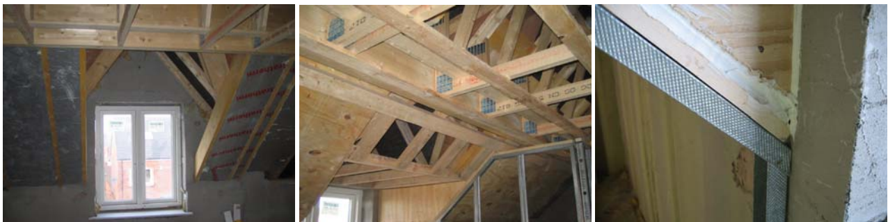
Figure 88. Dormer window in Redrow house types with plywood sheathing on the dormer cheeks sealed prior to dry-lining.
