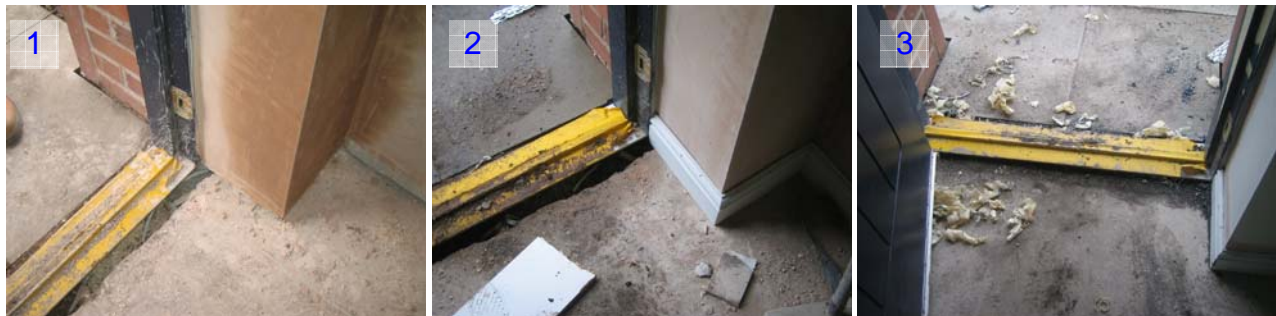
Figure 40. The front door threshold in plot R117.
