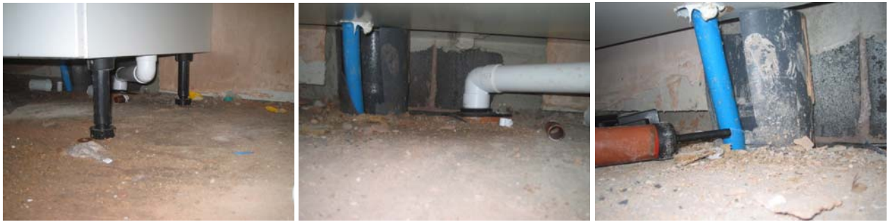
Figure 37. Utility room water supply and waste pipes in plot B119
