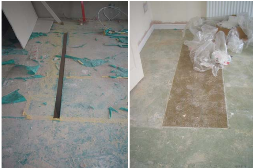
Figure 109. Holes cut and then repaired in a first floor in order to pass plasterboards to upper floors.
