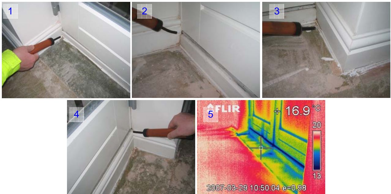
Figure 14. Infiltration at patio doors installed on intermediate floors in plot R110 with joists running parallel to the external wall (1, 2 & 3) and plot R111 with joists running perpendicular to the external wall (4 & 5).
