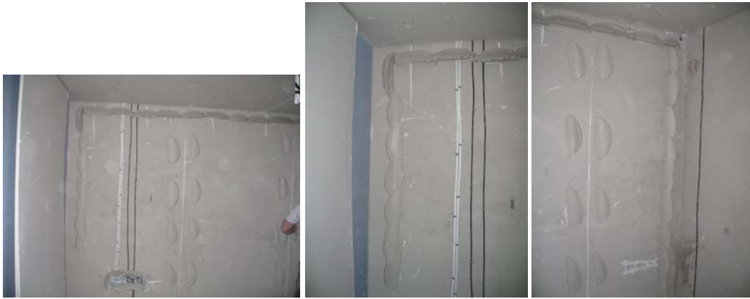
Figure 50. Continuous ribbons of plasterboard adhesive on an external wall in plot R116.
