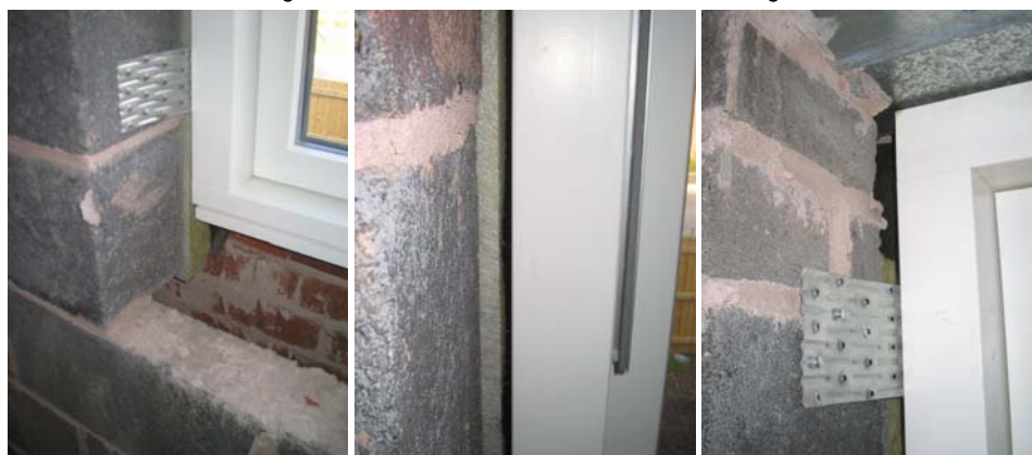
Figure 98. Incorrect window formers found in plot B121 and acoustic cavity barrier used instead of the proprietary formers in plot B117.
