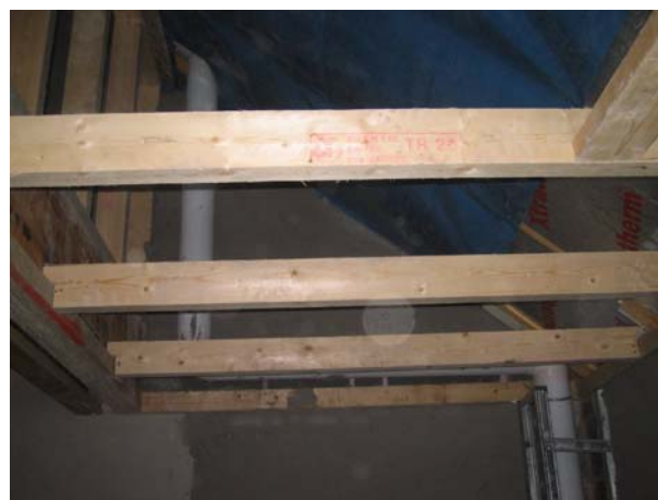
Figure 87. The service void in the 1 st floor bedroom in plot R117 entering the void between the eaves and 2 nd floor knee wall, and gap at the junction with the 1 st floor.
