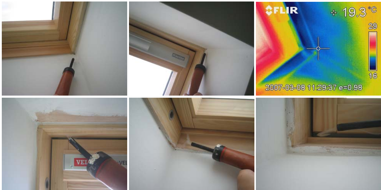
Figure 22. Air leakage at the rooflights, around the frames in plots R116 and R117 and between the rooflights and frames in plots B120 and B121.
