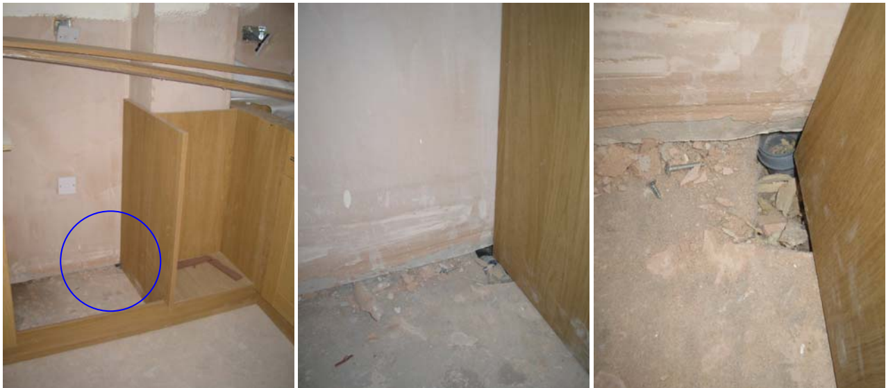
Figure 38. The gap in the screed at the base of the service void in plot B120 left which should have been filled prior to installation of the kitchen units.
