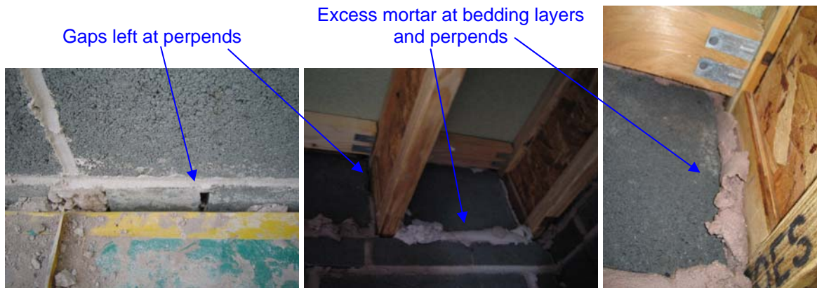
Figure 54. Gaps at perpend and excessive mortar around built-in joists creating difficulties for sealing.
