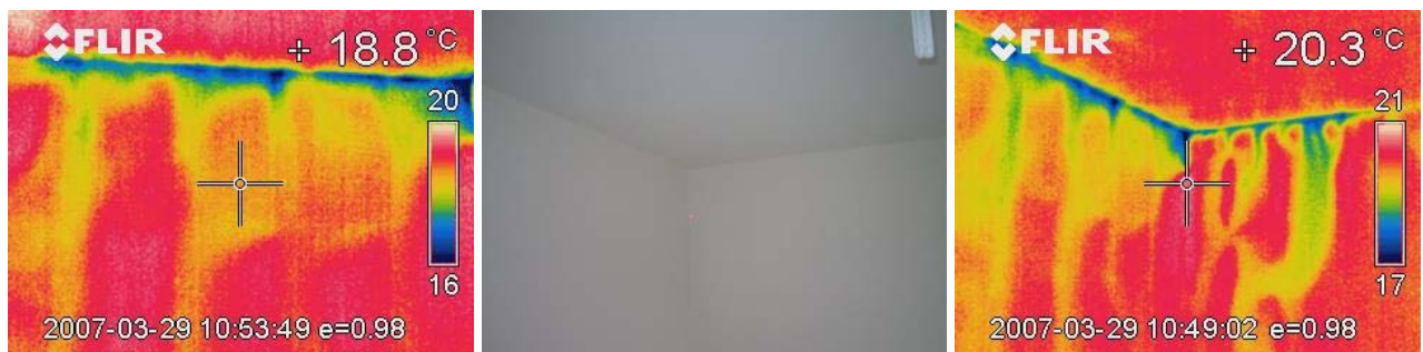
Figure 33. Infiltration at the tops of partition walls in plot 111 on either side of the 2 nd floor bathroom, the pattern of the studwork is visible and contrasts with the airflow around the plasterboard dabs on an adjacent external wall.
