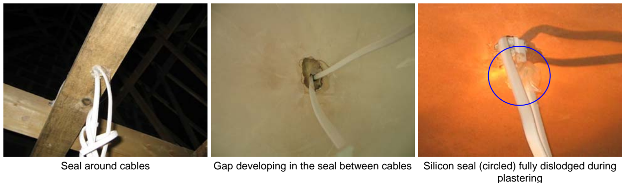
Figure 77. Dislodging of seals at electrical service penetrations.
