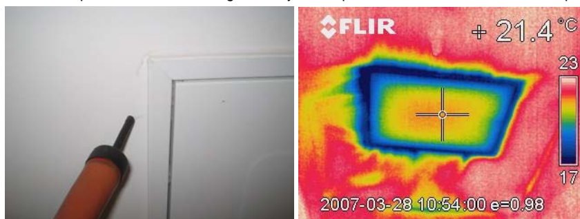
The photograph of the loft hatch in plot R110 indicates some air leakage, the IR image of the same detail provides further illustration of the extent of the problem.
