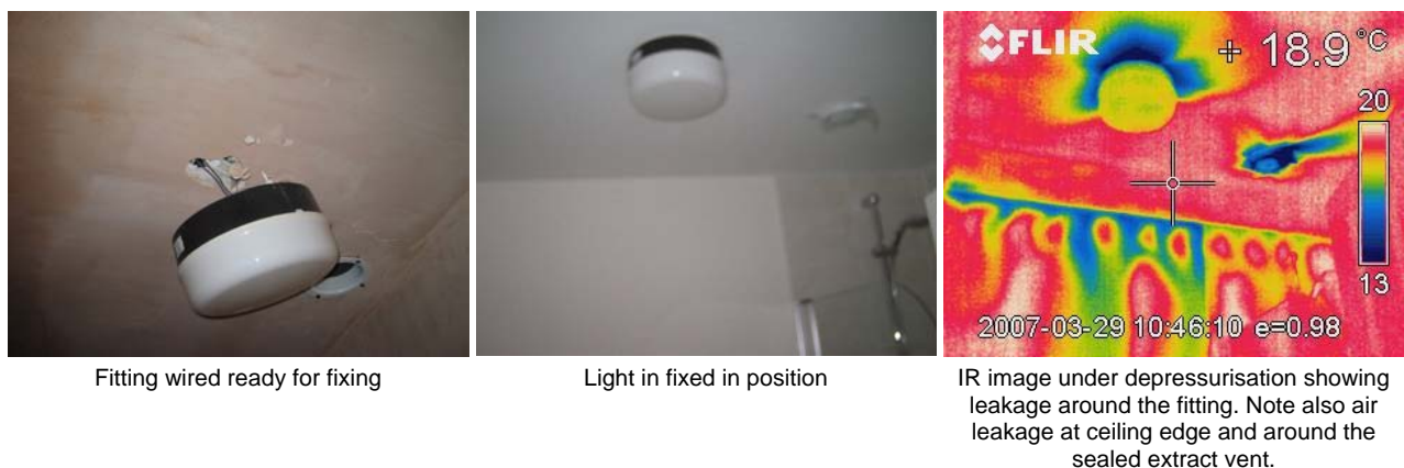
Figure 78. Air leakage around the ceiling light fitting in the 2 nd floor bathroom of plot R111
