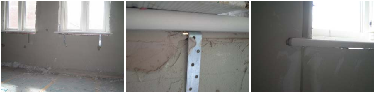
Figure 61. Daylight visible through gaps beneath the window sills in plot B121; after sill board installation, after patching and after dry-lining.
