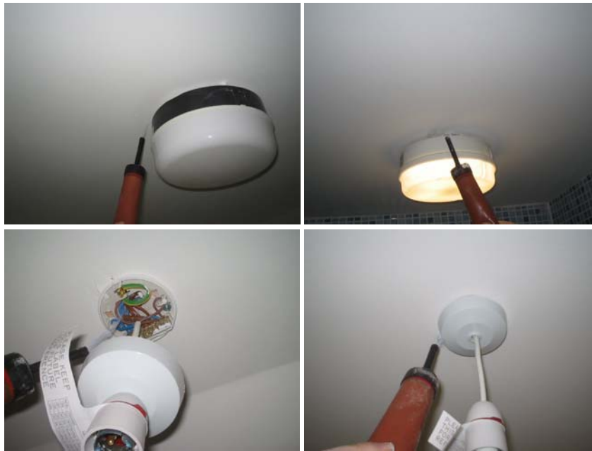
Figure 20. Air leakage into the loft around the 2 nd floor bathroom lights in plots R110 and B119, and at standard ceiling-mounted fixings for lights in top floor bedrooms in plots B121 and B119.
