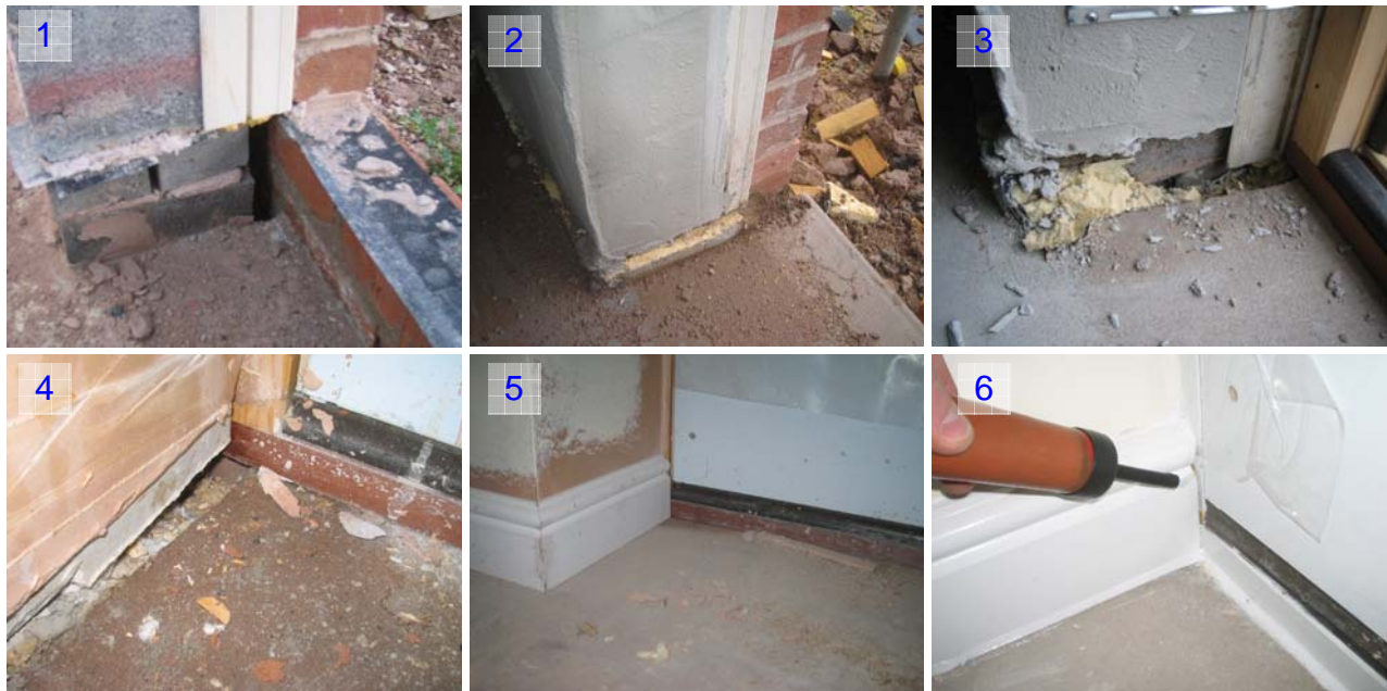
Figure 39. The build sequence of the threshold for Bryant, leaving the potential for air transfer between the cavity and the void behind the skirting.
