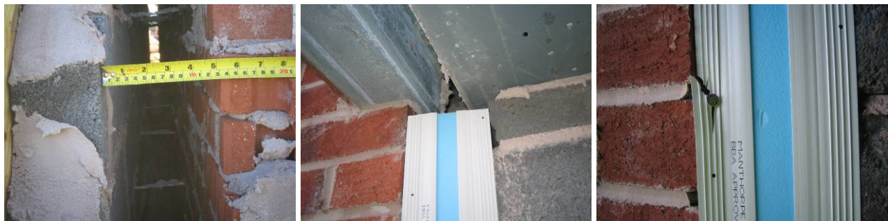
Figure 105. Variations in cavity width in plot R110 from 10% narrower than specified, to 10% larger where the originally specified cavity closers had to be replaced.
