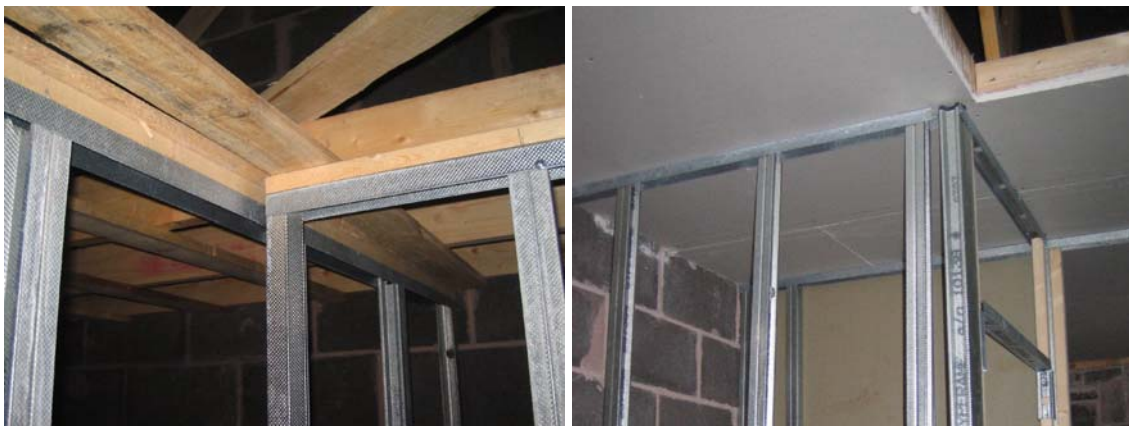
Figure 4. The potential for air leakage directly into the loft via top floor partition walls in Redrow plot R111 compared to Bryant plot B116 with a full ceiling installed before the partitioning.
