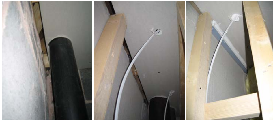
Figure 82. Sealing at the service void head in the bathroom of plot B117.
