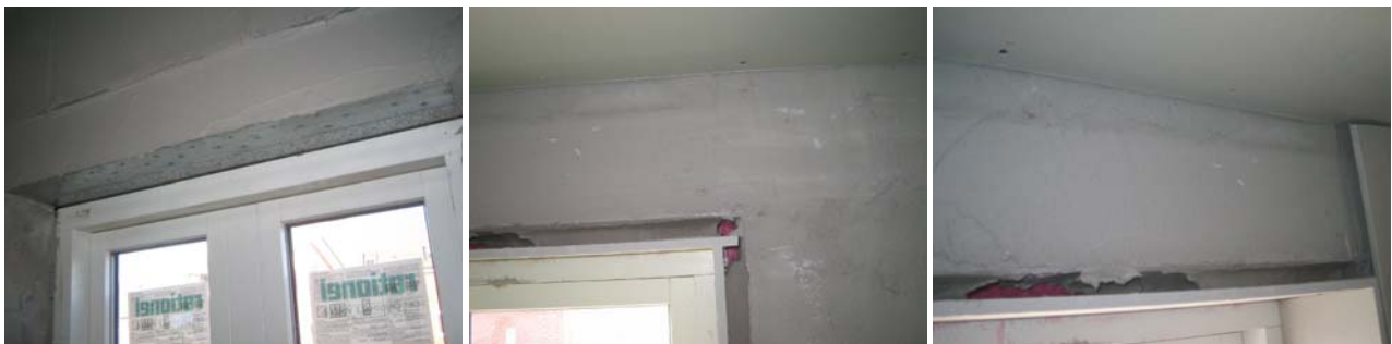
Figure 62. Window heads with no parging to the underside of the lintel and with large spaces left between adhesive dabs bonding the head liner.
