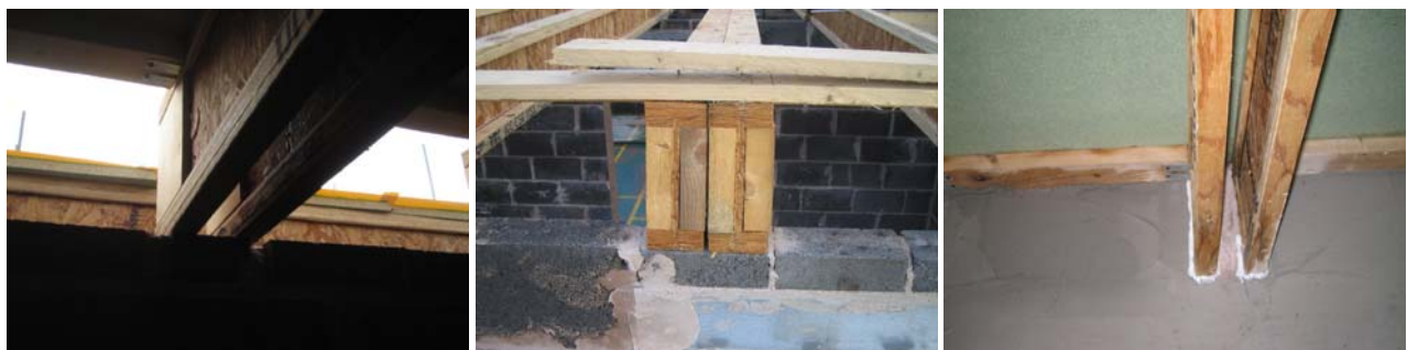
Figure 58. Double I-beams in plot B120 with a small gap between, giving limited access to gap between the joists.
