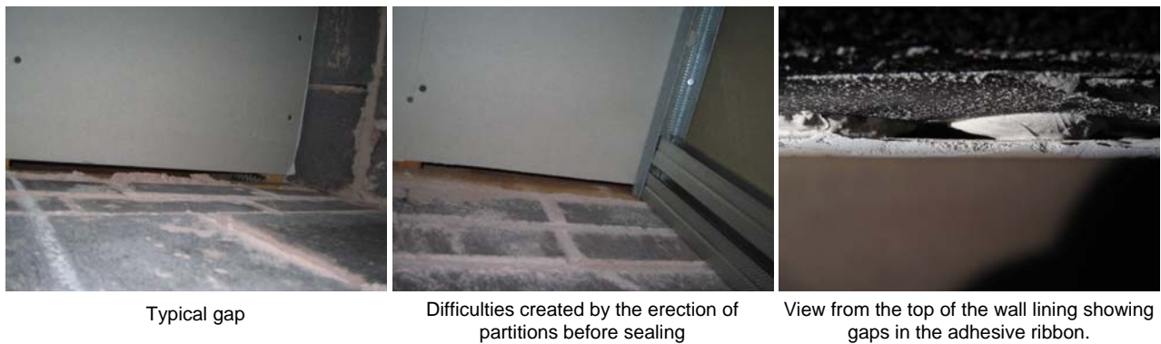
Figure 74. Gaps around the edge of ceiling boards which were not adequately sealed when the parging coat and wall dry-lining were applied.
