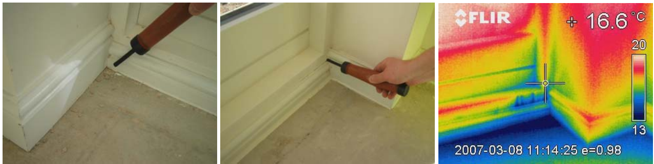
Figure 12. Air leakage at the gallery window “thresholds” in plots R116 and R117, the thermal image showing infiltration in plot R117 at this detail
