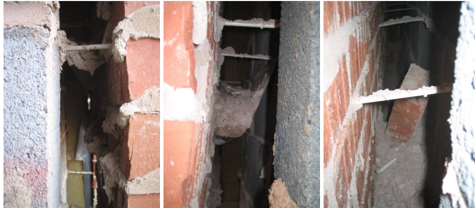
Mortar snots affecting the placing of the vertical cavity barrier in plot B116.
