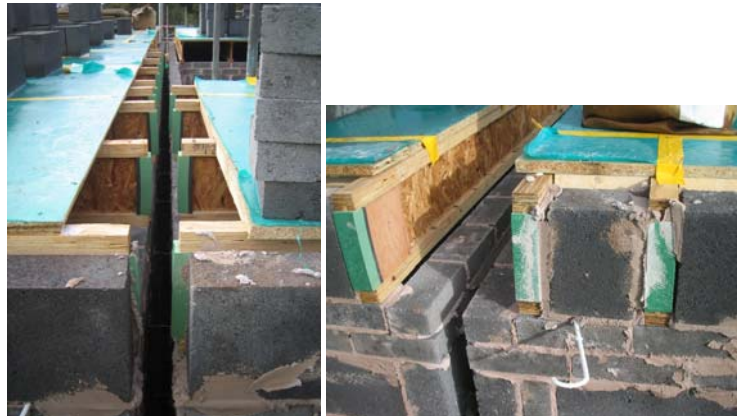
Figure 52. Difficulties of gaining access to construct well sealed blockwork in intermediate floor space.
