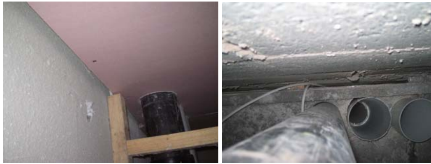
Figure 81. The junction of the wall and ceiling inside the service void in the rear en-suite bathroom of plot B121.
