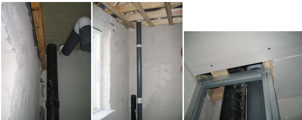
Figure 84. The service void in the front of the Mendip house type, from the 1 st floor en-suite, through the 2 nd floor front bedroom into the loft in plots R110 and R111.
