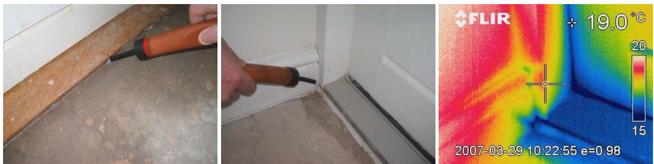
Figure 13. Direct air leakage at patio doors thresholds in various plots.
