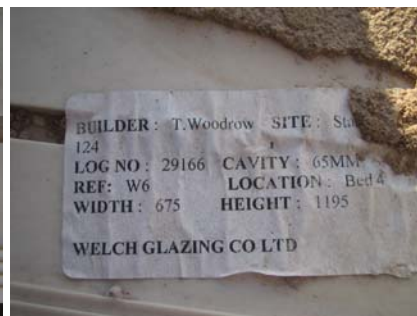
Window former installed in the wrong plot and wrong room
