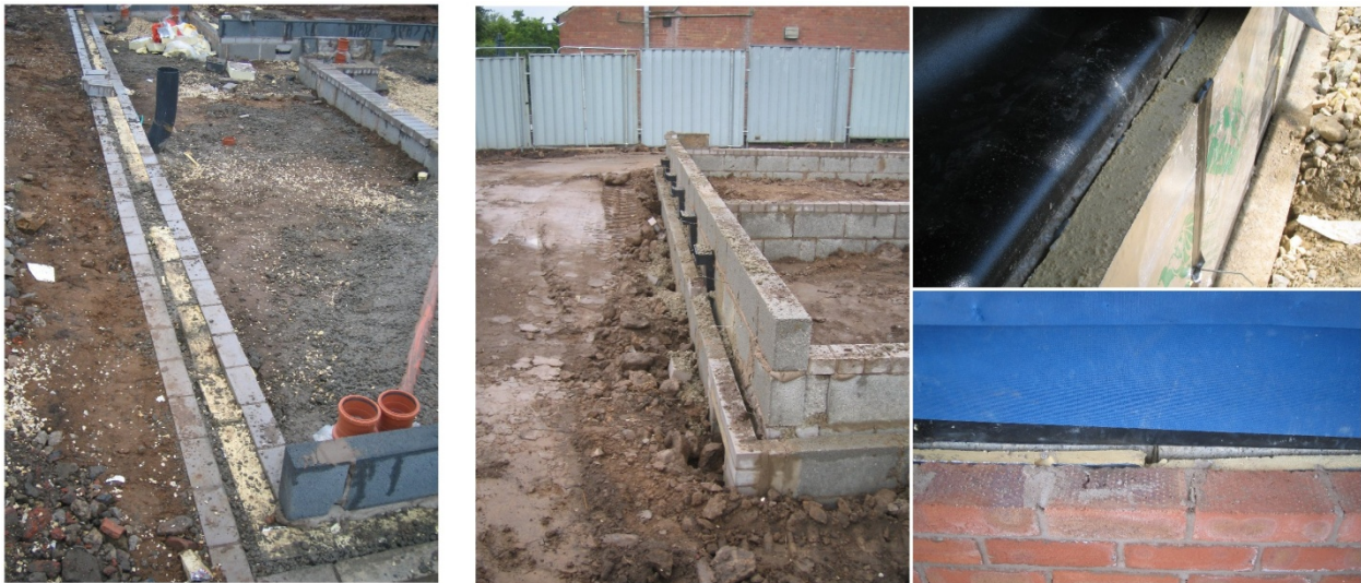
Figure 3 Perimeter insulation below floor level in the masonry prototype, and at various stages on the SIPs prototype.
