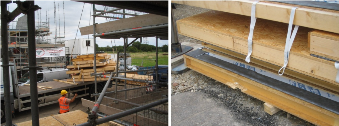
Figure 8 Unloading of the SIPs panels and the resulting damaged panel.
