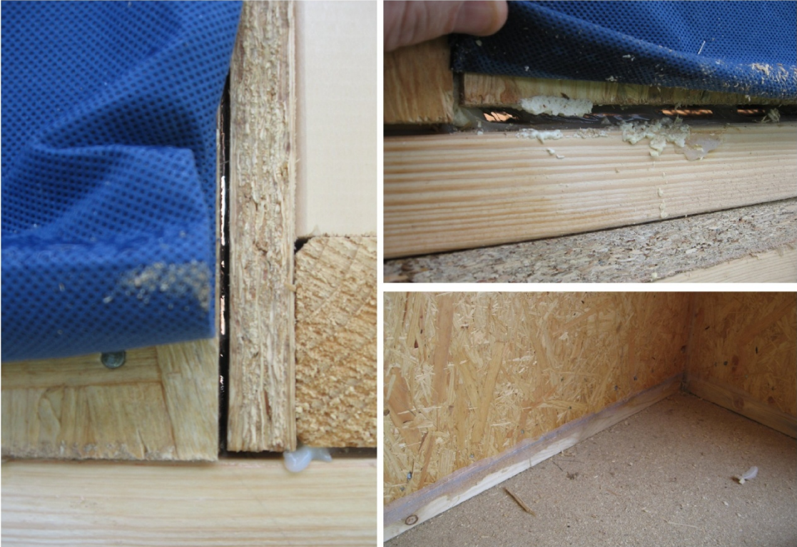
Figure 7 Gaps observed between SIPs panels during construction were sealed using a silicone mastic as construction progressed.
