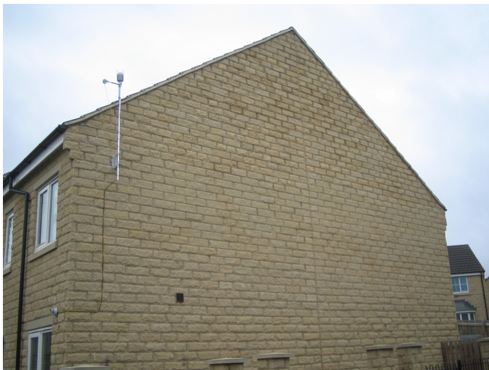
Figure 4 Coeating test weather station installed on a gable wall.
