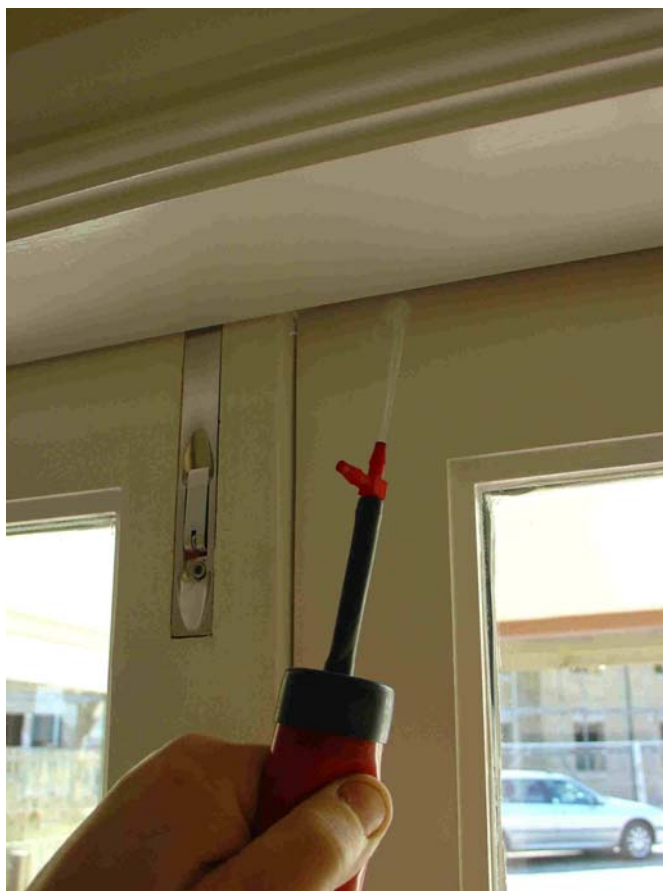
Figure 18 - Leak at Warped Sun-space Doors (Plot 16)
