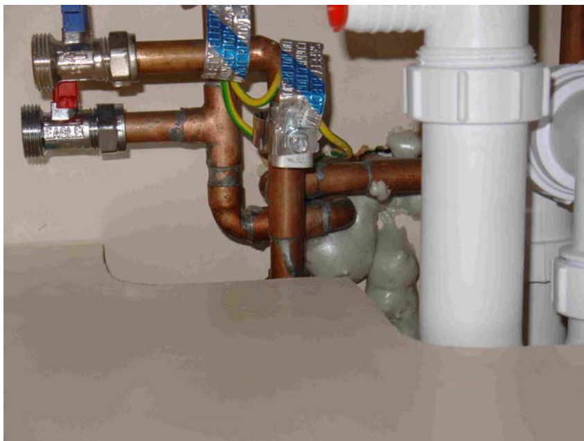
Figure 28 - Use of Expanding Foam to Seal Service Penetrations in Kitchen of Unit 4
