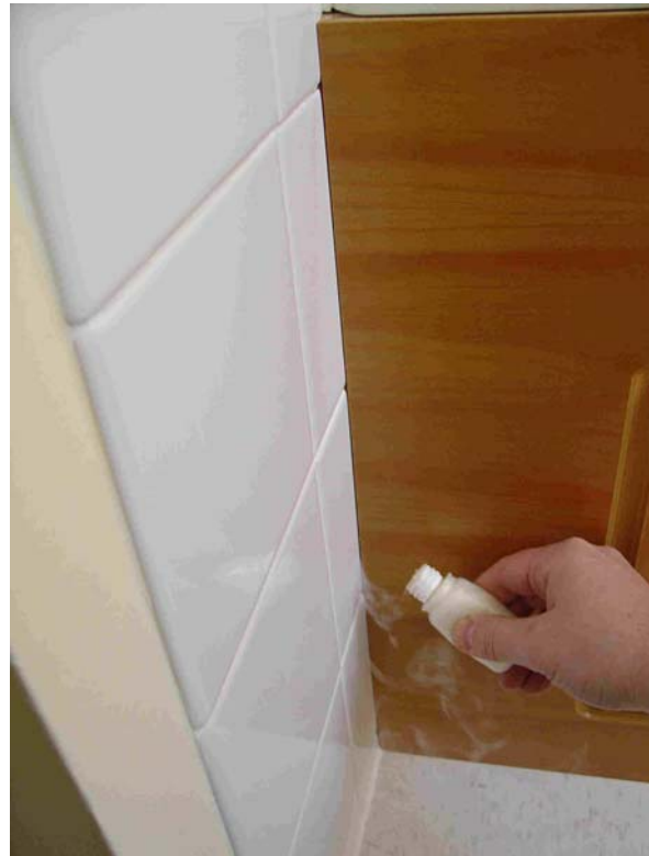
Figure 15 - Leak around Bath Panel (Plot 16)
