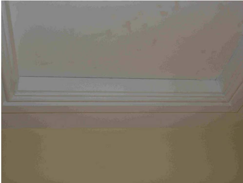
Figure 24 - Gap around Loft Hatch (Plot 16)
