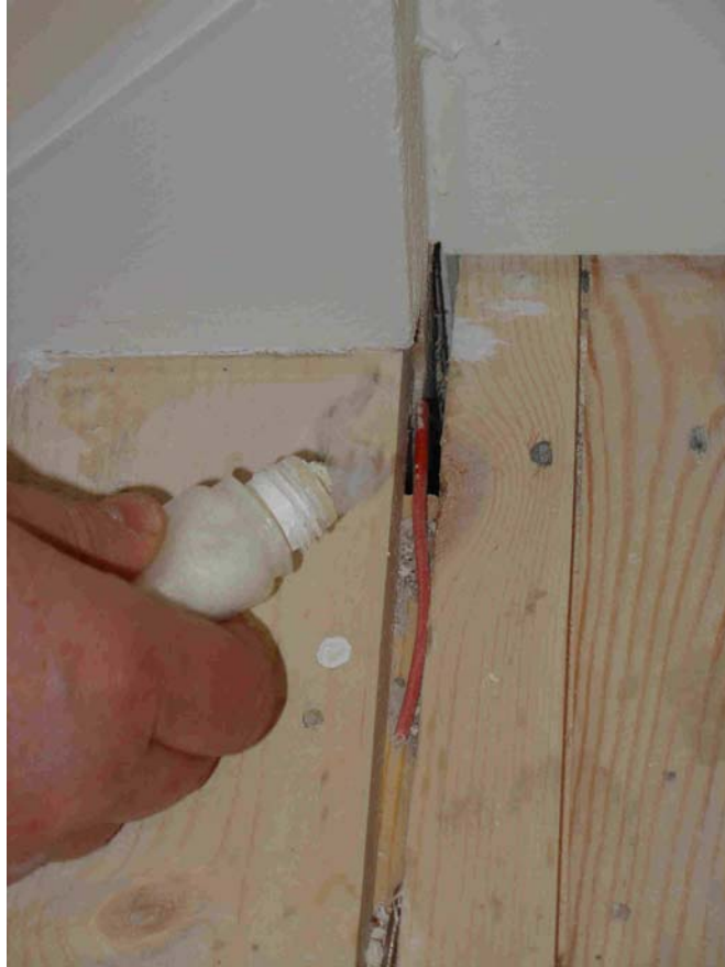
Figure 20 - Leak at Gap in Flooring (Plot 4)
