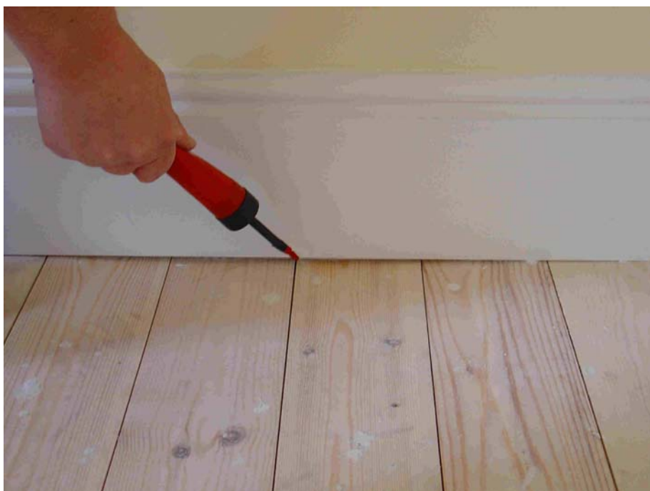
Figure 19 - Leak at Gap between Skirting Board & Floor (Plot 4)
