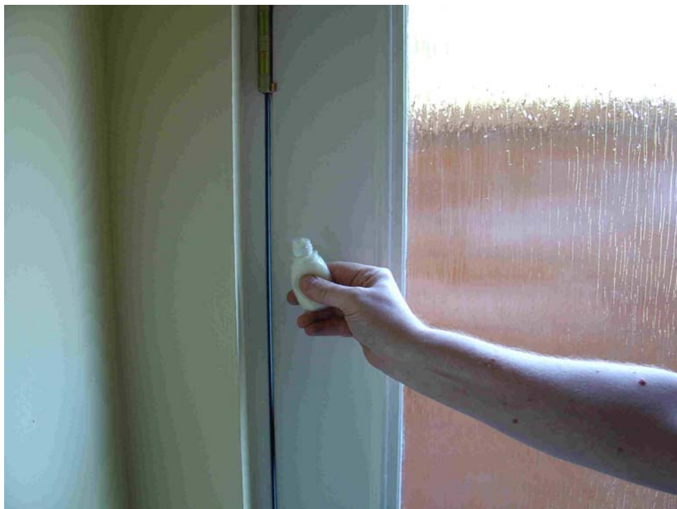
Figure 17 - Leak around Back Door Frame with Smoke Shown Flowing Outside (Plot 16)
