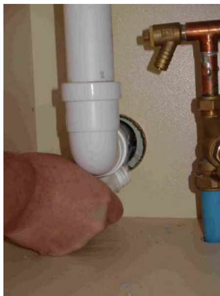
Figure 13 - Leak around Sink Outlet Pipe Penetration (Plot 16 kitchen)
