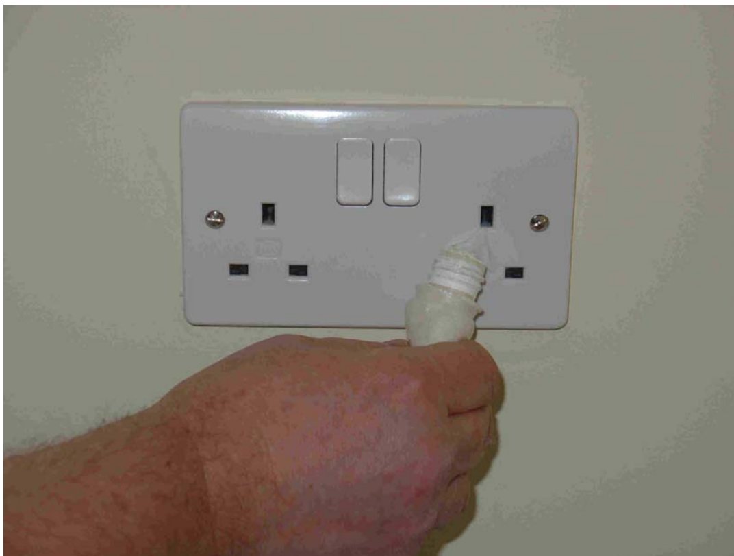
Figure 23 - Leak through Electrical Socket (Plot 18)
