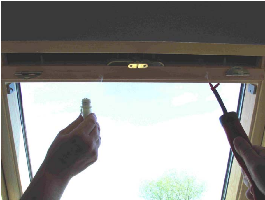
Figure 26 - Leak through Missing Velux Trickle Vent/Handle (Plot 17)
