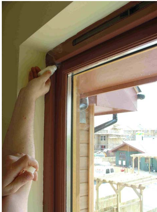
Figure 25 - Leak around Window Frame in Bedroom with Smoke Flowing Outside (Plot 4)
