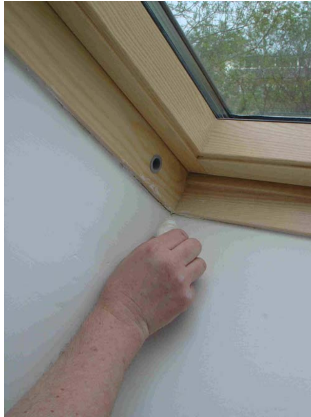
Figure 16 - Leak at Gap between Velux Frame and Wall (Plot 4)
