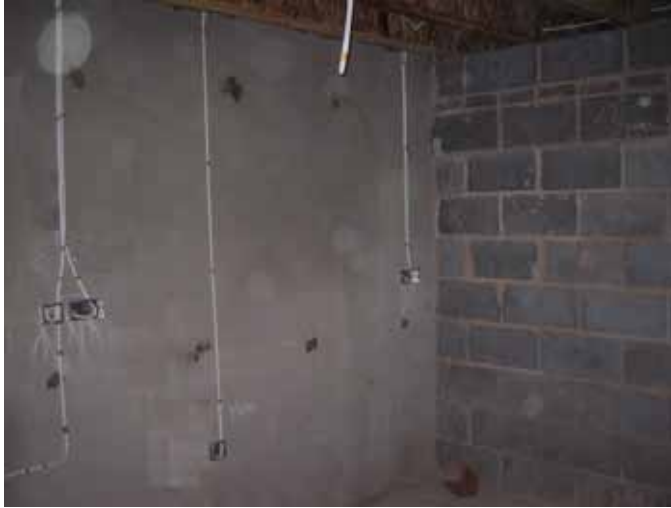
Figure 9: Parging showing insulation drill holes filled with mortar.
