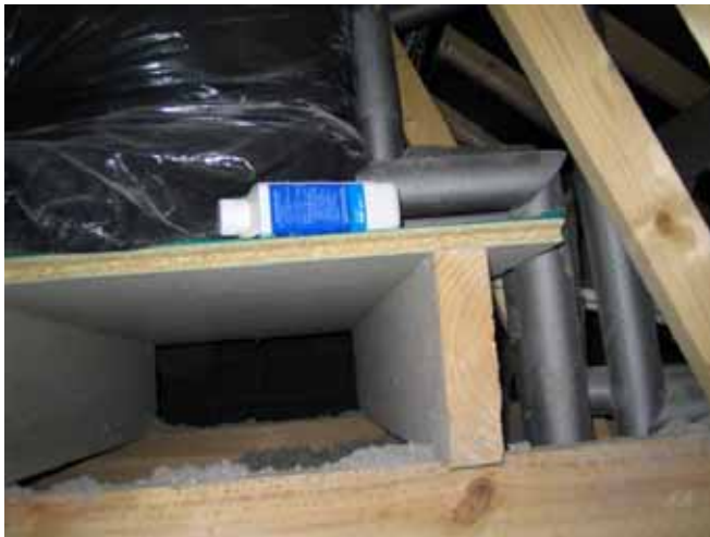
Figure 16: Unvented system. Feed and expansion tank in loft space showing platform and additional insulation required.
