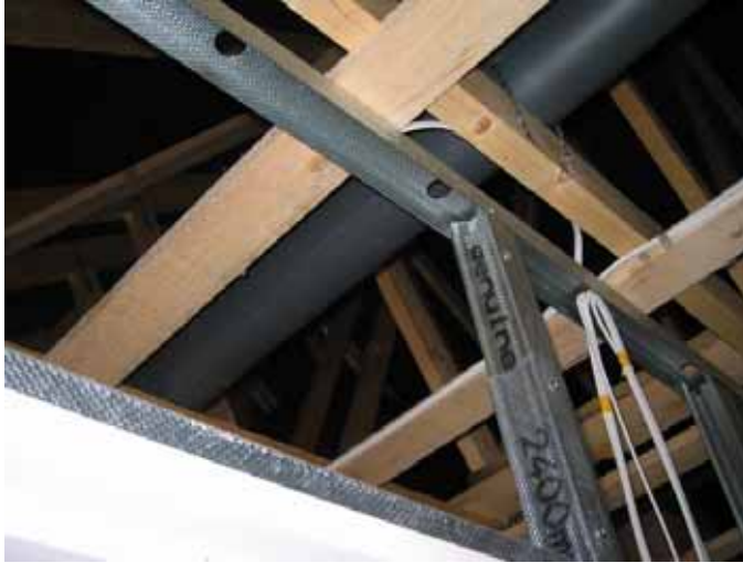
Figure 12: Metal studwork showing potential air leakage paths through pre-cut service access holes in head plate.
