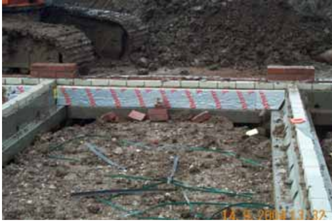
Figure 3: Insulation problems around ringbeam foundation.
