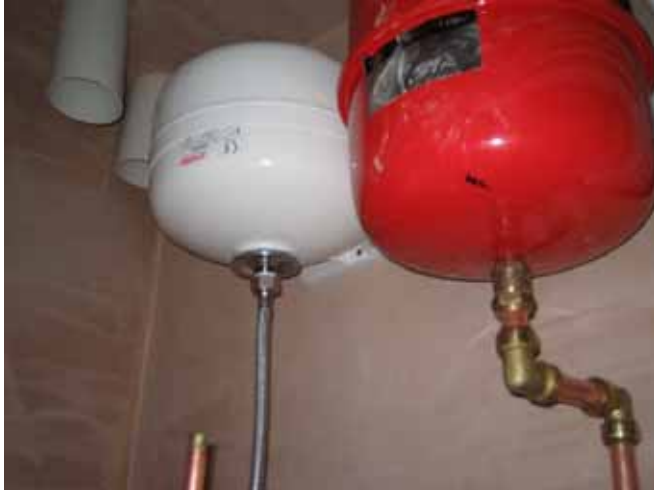
Figure 17: Vented system. Pressure vessels in heated envelope of building.
