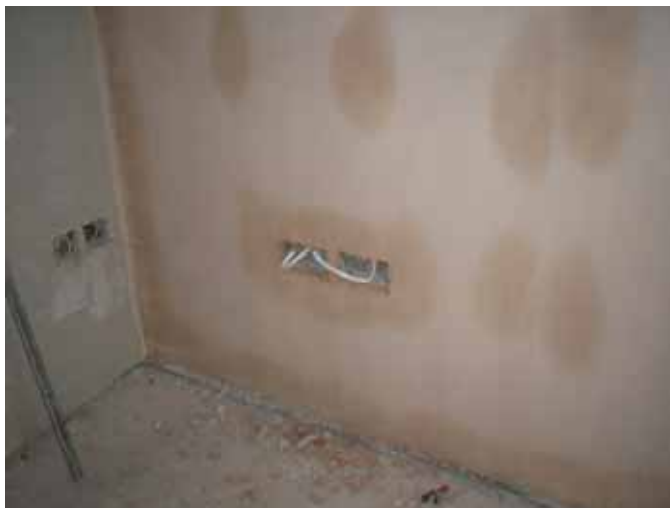
Figure 13: Plasterboarding showing continuous ribbons of bonding at perimeter and around electrical boxes.
