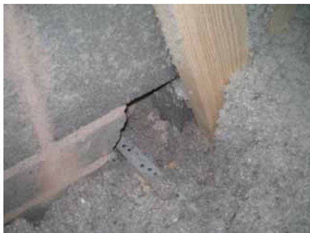
Figure 52 – Gap in Party Wall in Loft for Restraint Strap - Redrow
