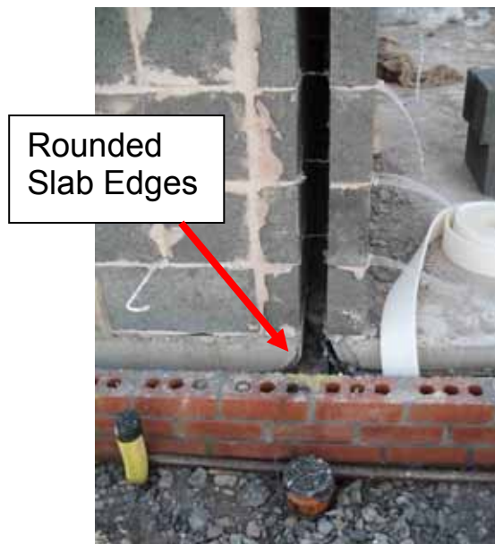
Figure 56 – Imperfect Floor Slab Edges
