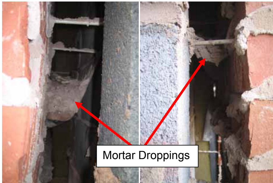
Figure 59 – Mortar Build up on Cavity Tray
