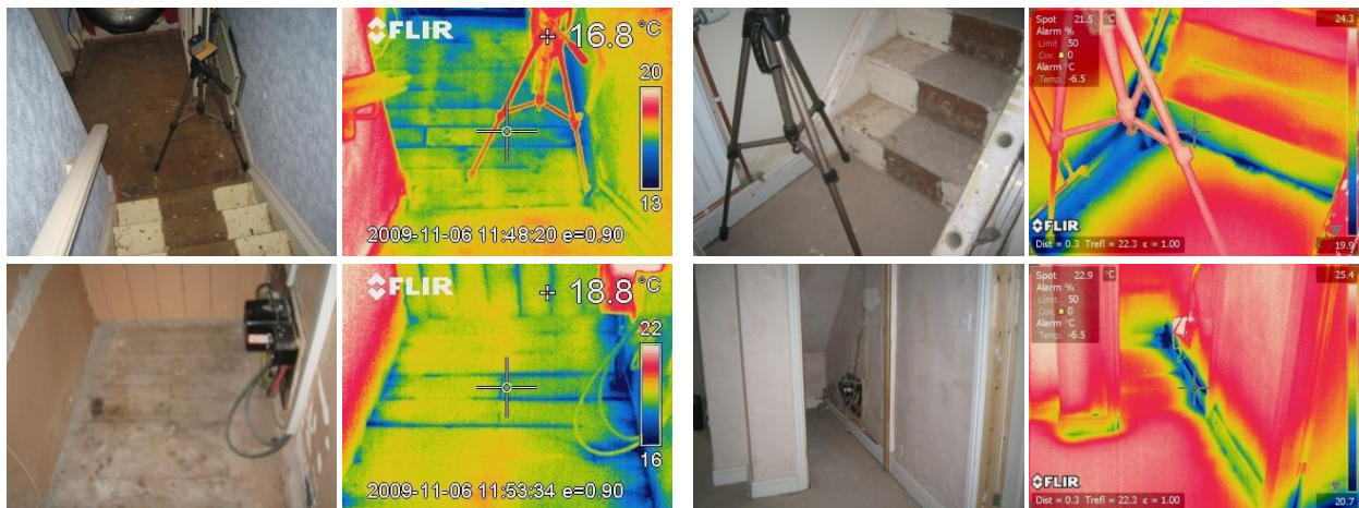
Figure 39 The hall and cupboard under the stairs, under depressurisation, showing the difference between the suspended timber ground floor and the replacement insulated solid concrete ground floor.
