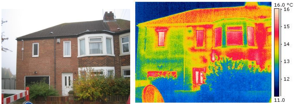
Figure 4 Front elevation during coheating test 1, 27-Oct-09, prior to cavity wall insulation installation.
