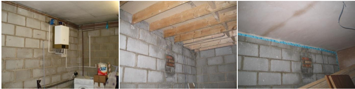
Figure 15 The boiler and associated pipework were removed and a new intermediate floor constructed over the garage.
