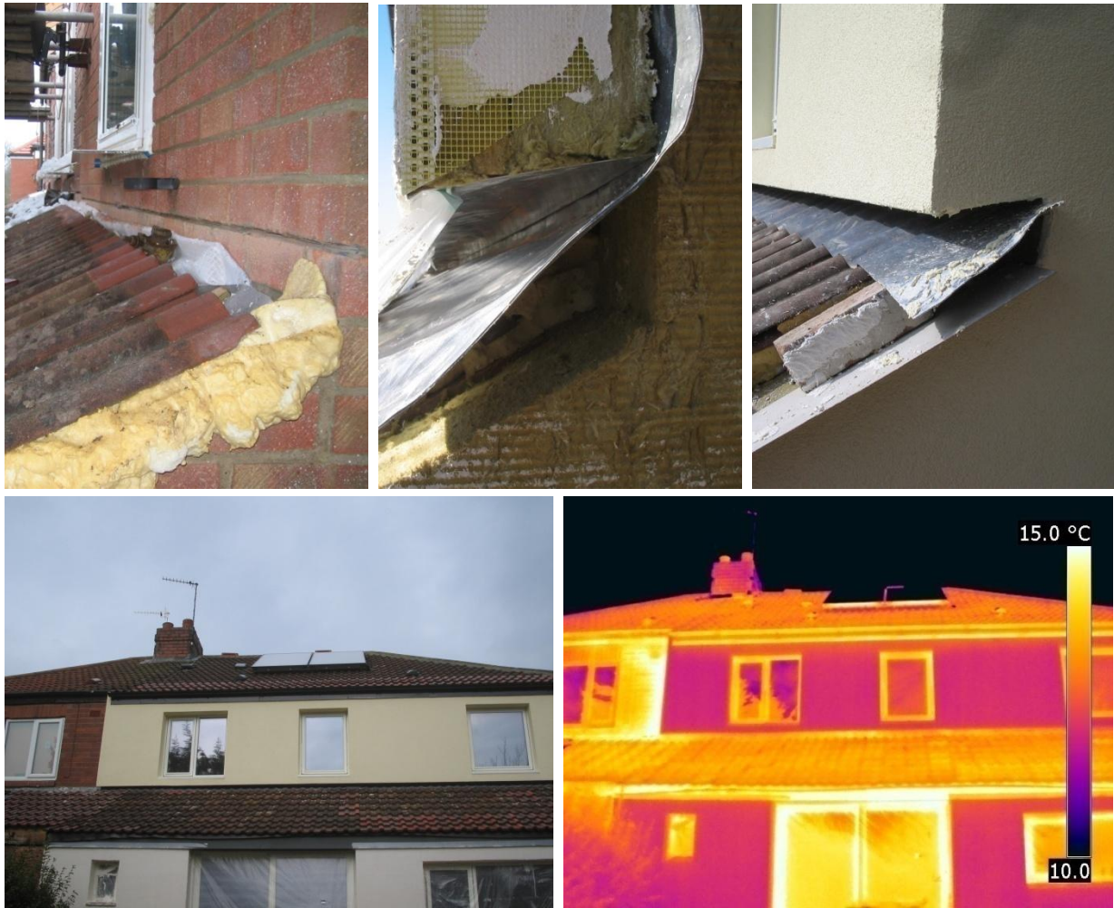
Figure 25 Junction of EWI with the rear extension roof at various stages of construction, and a thermal image of the completed detail captured during the 3 rd coheating test.
