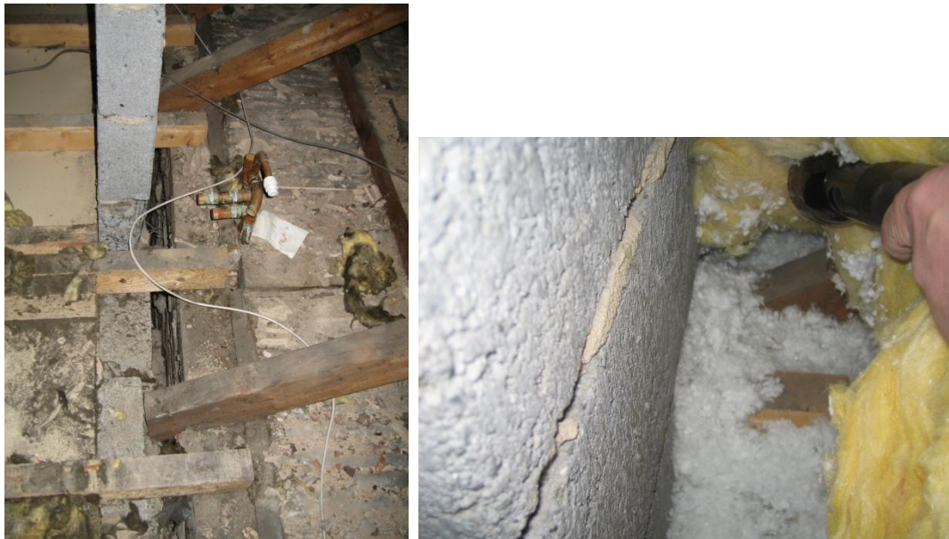
Figure 11 The top of the internal cavity wall with the old insulation removed and with the cavity filled and new loft insulation laid.
