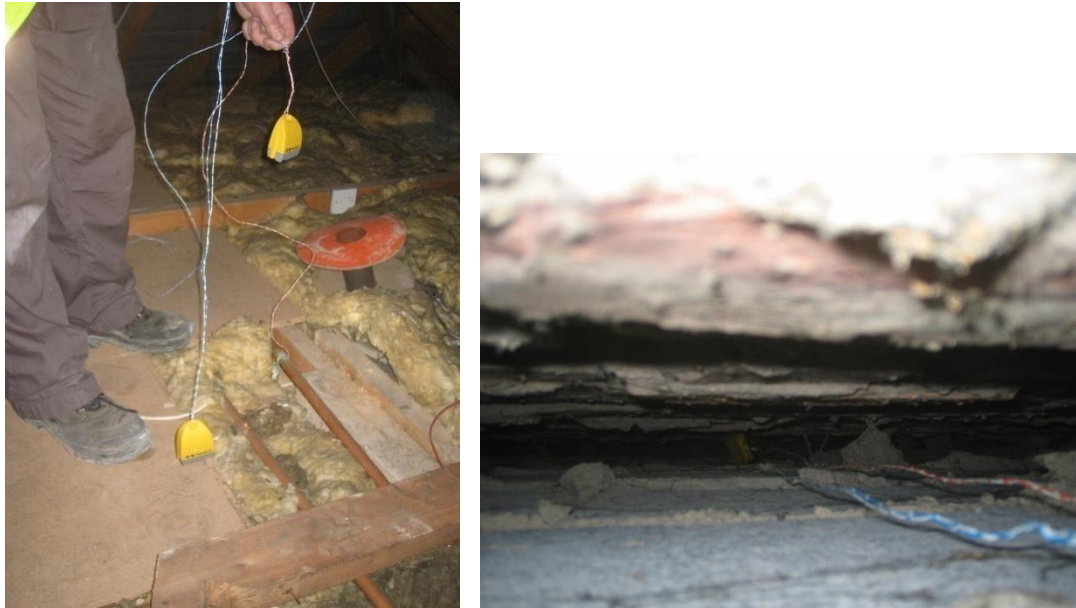
Figure 60 TinyTag data-loggers, suspended on wires and dropped down the internal cavity walls to investigate the potential thermal bypass.
