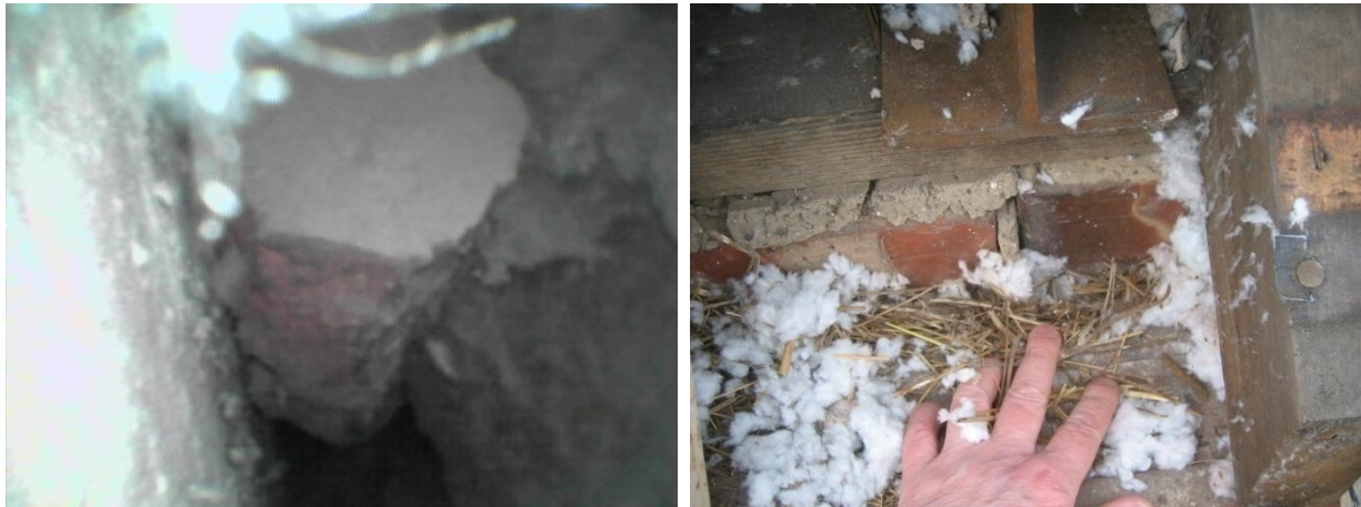
Figure 8 Debris in the cavity wall included masonry detritus and bird nests.
