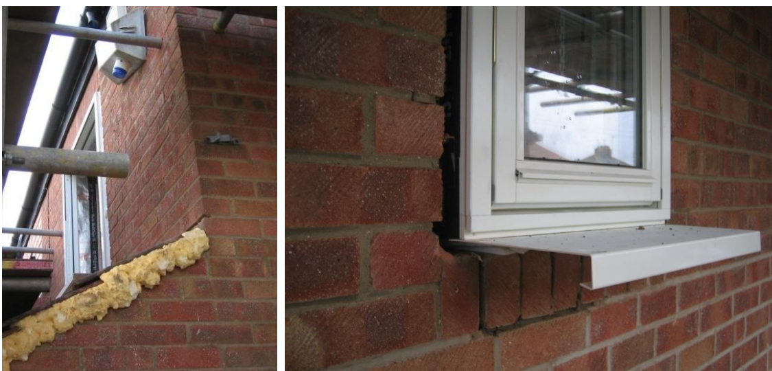
Figure 32 Rear and front elevation window frame positioning, showing potential for overlap with the EWI.
