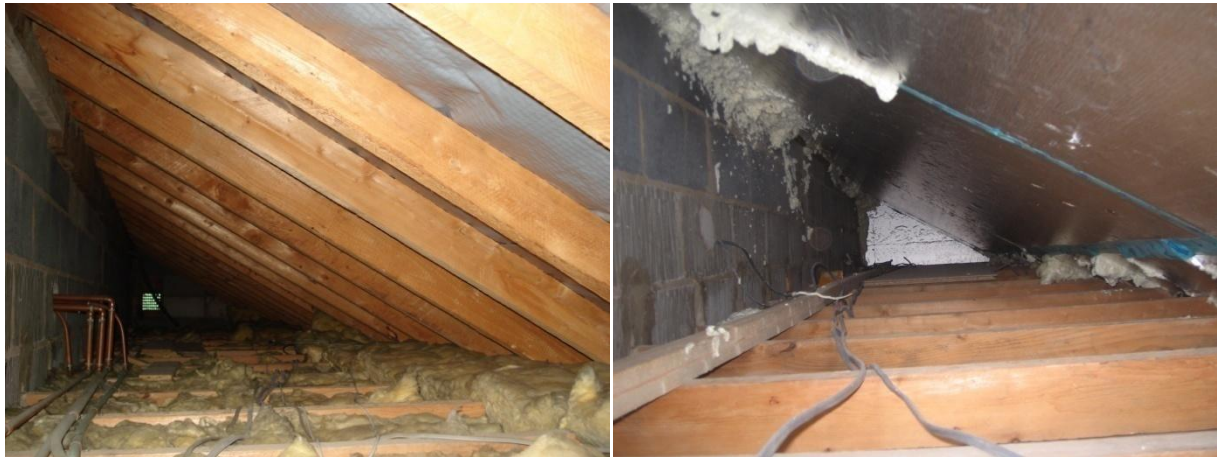
Figure 12 The rear extension insulation was relocated from mineral wool between the joists to phenolic foam beneath the rafters.
