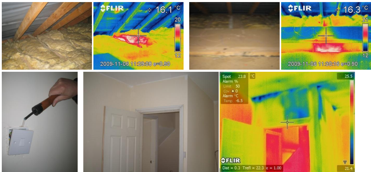
Figure 42 Hot air escaping through the partition wall heads into the loft in the 2 nd pressurisation test in November 2009 under dwelling pressurisation. And in March 2010, air leakage into the 1 st floor partition wall voids; via an electrical pattrass under dwelling pressurisation and from the roof space under depressurisation.
