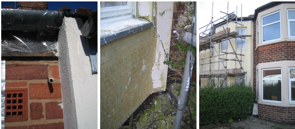
Figure 26 The edge detail of the EWI at the party wall junction at the rear and front elevations.
