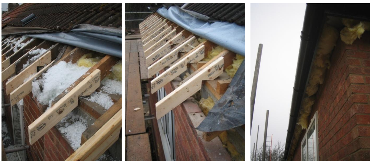
Figure 28 Eaves extensions to the main roof at the rear and side elevations under construction, and with the roof extension completed prior to the EWI installation.
