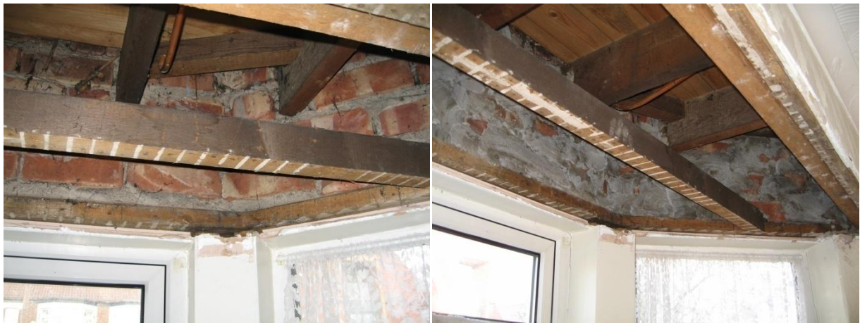
Figure 19 Void above the living room bay window re-pointed and sealed around the joists to reduce air leakage
