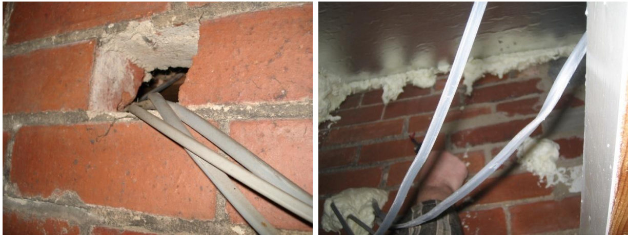
Figure 37 Gaps in the external wall in the rear extension loft space effectively became part of the air barrier and required sealing due to the movement of the air barrier from ceiling to rafter level in the rear ground floor extension.
