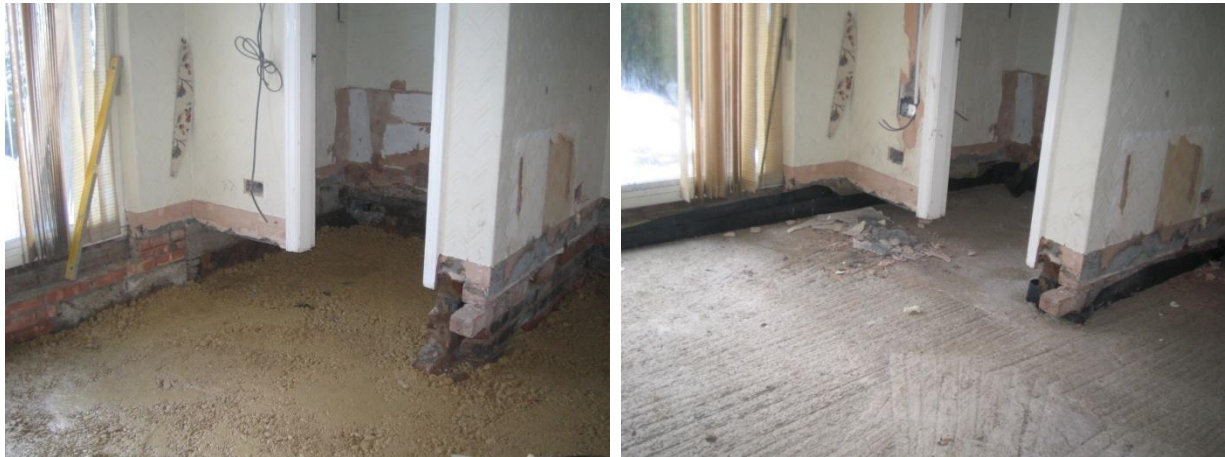
Figure 20 New ground floor construction in the dining area and previous downstairs WC.
