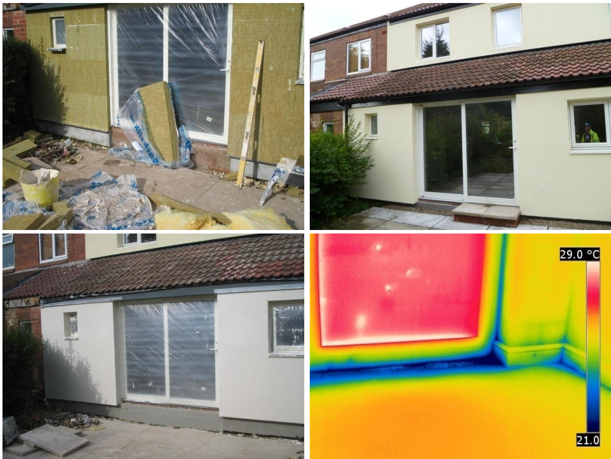
Figure 23 Patio door threshold during construction, on completion, and the external view and internal thermal image of the detail during the phase 3 coheating test.
