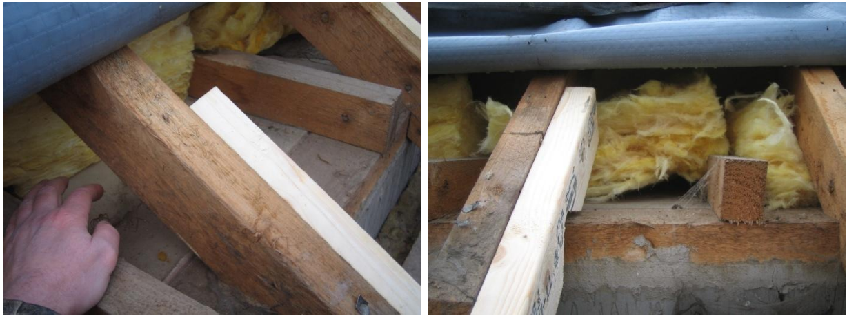
Figure 10 Loft insulation not extending fully into the eaves and air spaces around the insulation.
