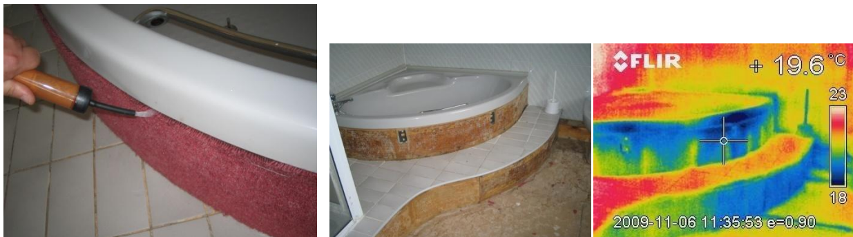
Figure 35 Air leakage around the bath in July 2009, using smoke detection under pressurisation, and cooler air being drawn in under depressurisation in November 2009.
