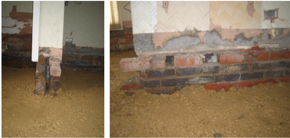
Figure 6 Removal of the original floors for Stage 2 renovation revealed the depth of penetration of the cavity wall fill.
