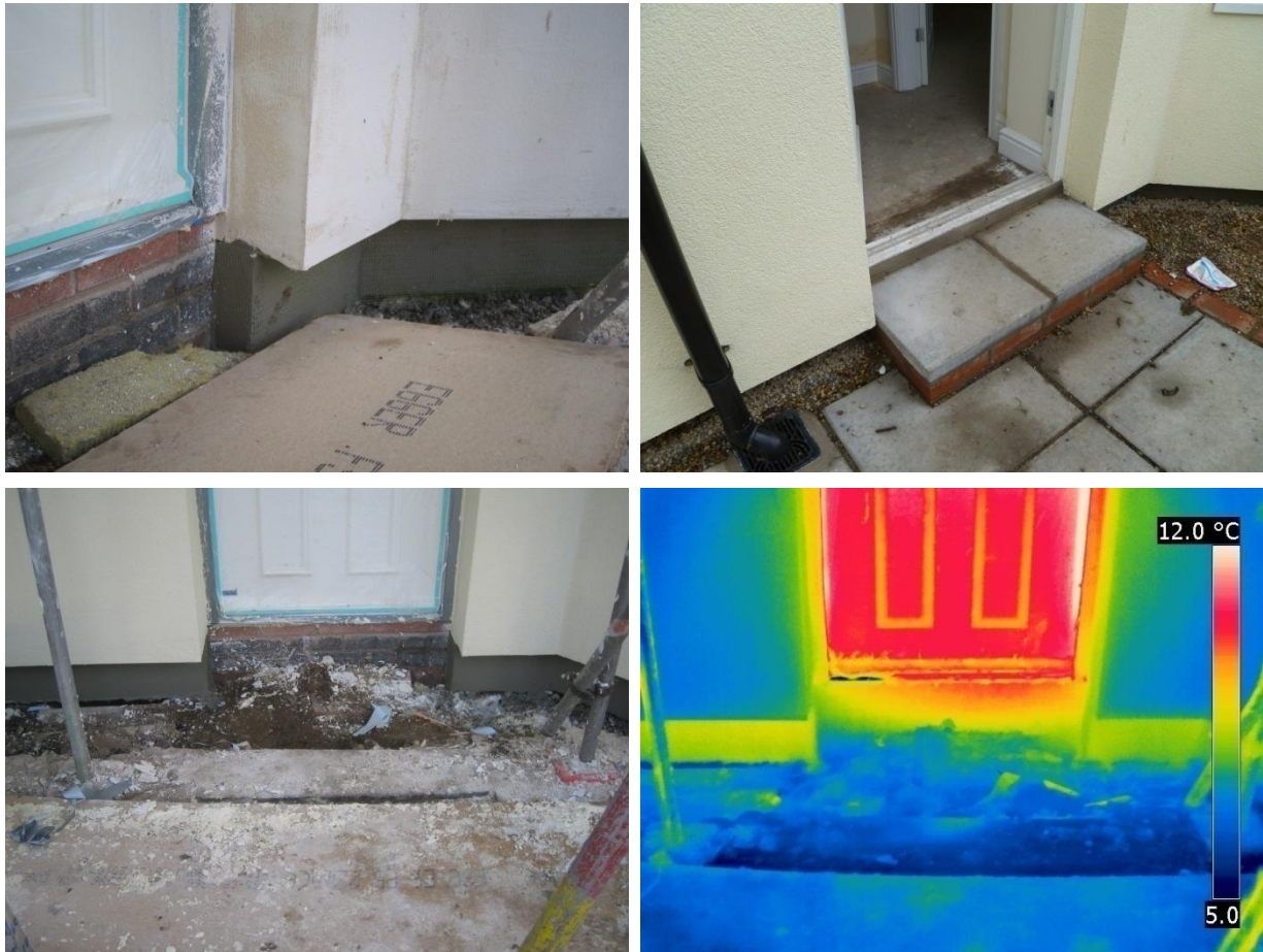
Figure 24 Front door threshold during construction, on completion, and the external view thermal image of the detail during the phase 3 coheating test.
