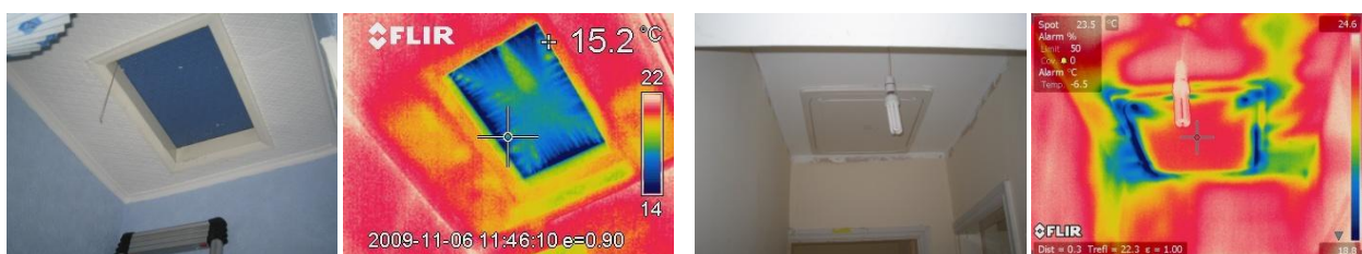
Figure 41 The original lofthatch into the main loft and the replacement, both under dwelling depressurisation.
