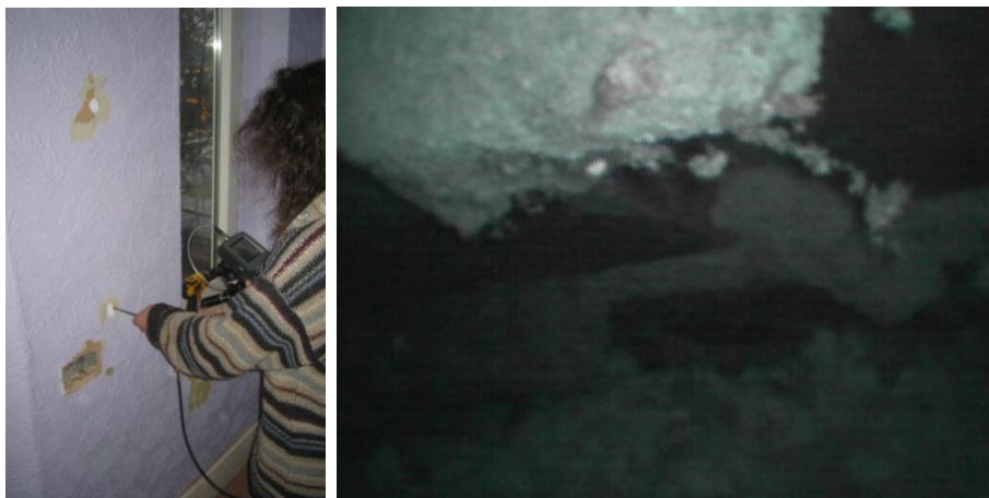
Figure 7 Boreoscope investigation of the external wall showing insulation clustered around the injection hole, but not filling the cavity.
