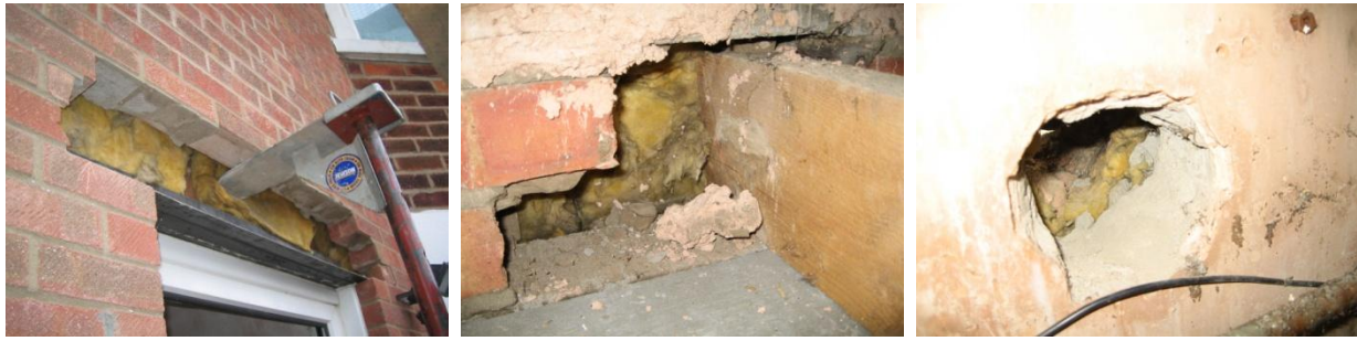
Figure 52 Cavity insulation at the front door, gable wall, and rear extensions wall was revealed during renovations works and shown to be thicker than originally estimated (photographs taken during relocation of the front door lintel, installation of the new extension floor and removal of the existing kitchen service penetrations).
