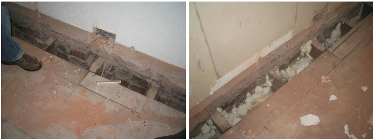
Figure 33 Rear wall of bedroom 2 before and after sealing work around the intermediate floor joists.
